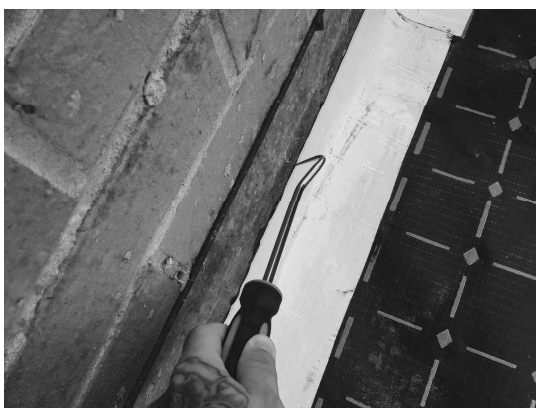
Probe test to retro fit detailing
