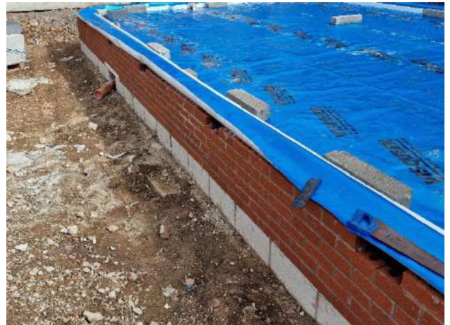
Figure 2 – Sufficient vents can be seen (every 2m).
