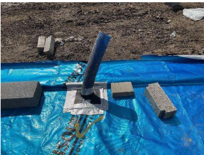
Figure 5 – Service entries patched correctly.
