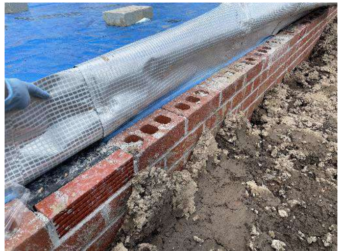
Figure 2 – Sufficient vents can be seen (every 2m).
