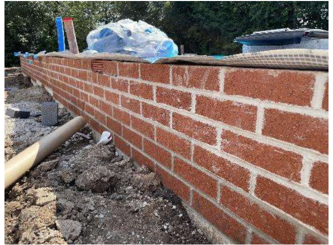
Figure 2 – Sufficient vents can be seen (every 2m).
