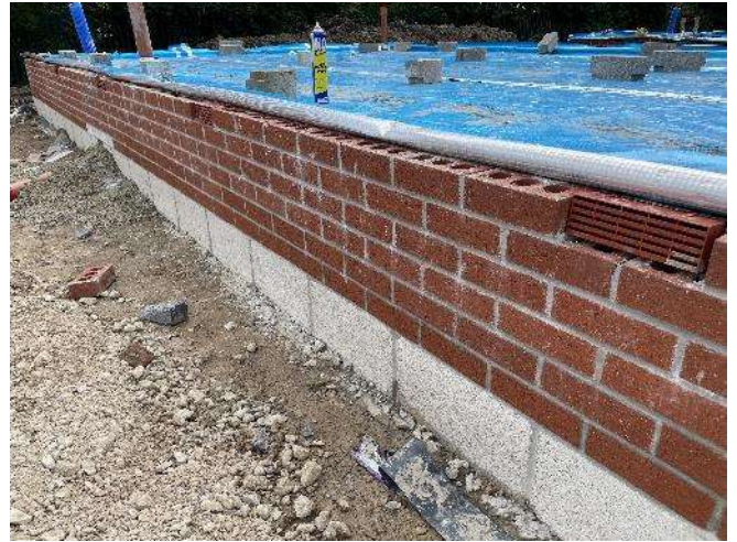
Figure 2 – Sufficient vents can be seen (every 2m).
