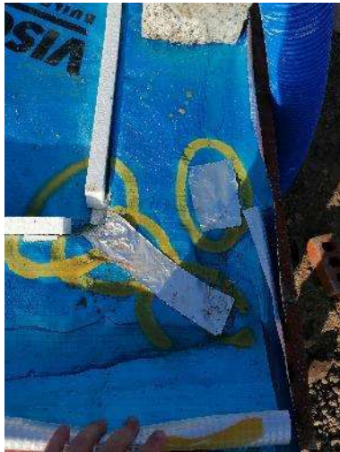
Figure 3 – Gaps in corners correctly sealed.
