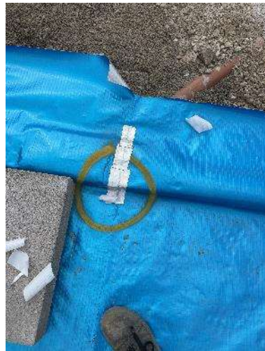
Figure 4 – Multiple gaps found in hand welded jointing were correctly patched.
