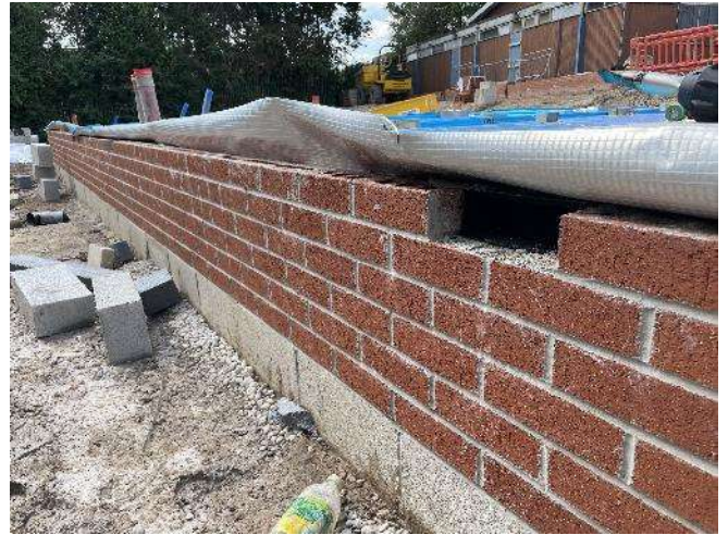
Figure 2 – Sufficient vents can be seen (every 2m) – air bricks to be added to periscopic vents.
