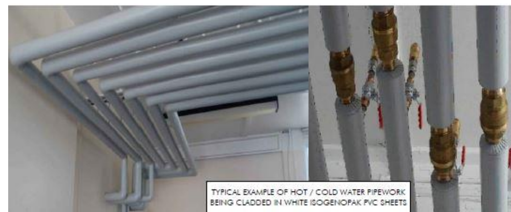
Fig 3: White pipe wrap for exposed water pipework
