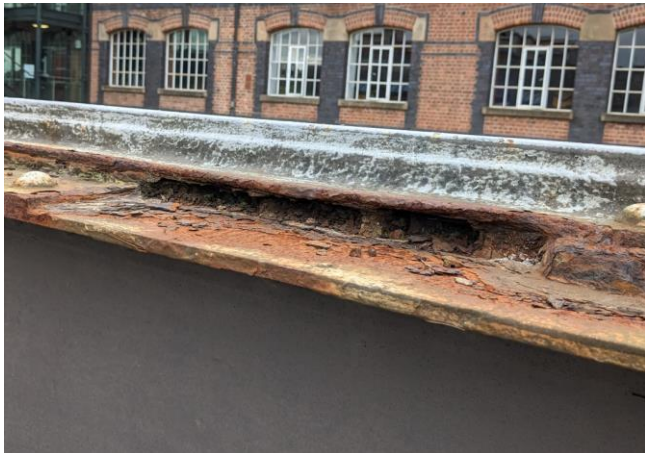
Figure 2-40 Moderate corrosion to top face Gantry beam
