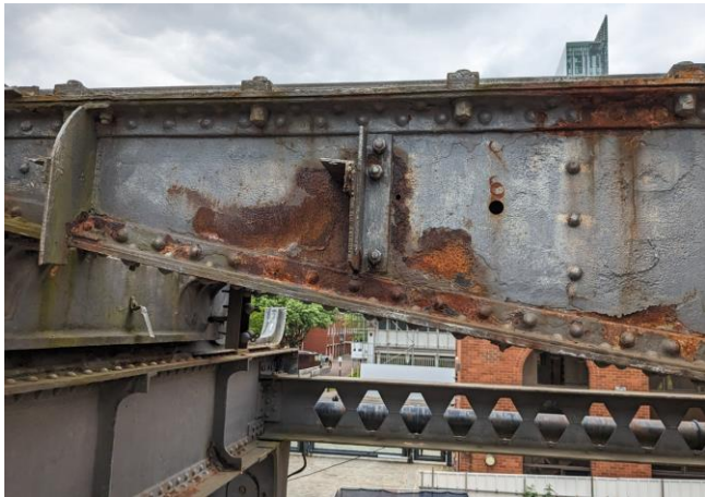
Figure 2-25 Corrosion to side face crane beam (eastern)
