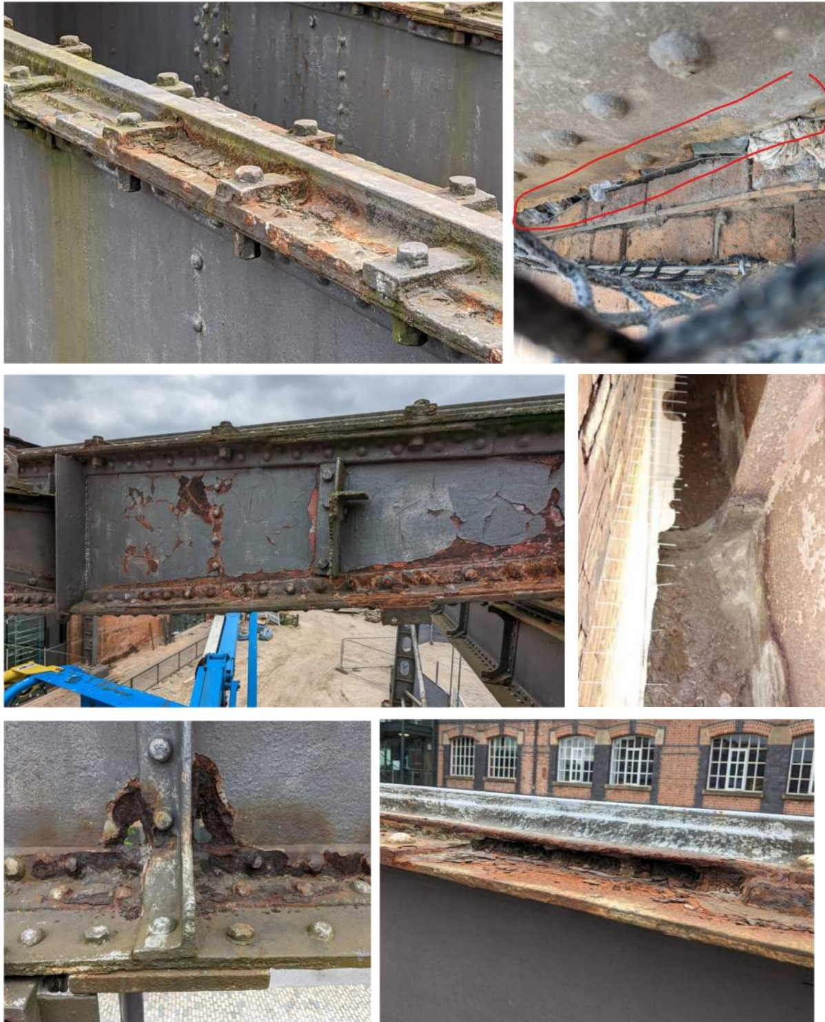
Figure 2-1 Typical examples of corrosion from structural survey
