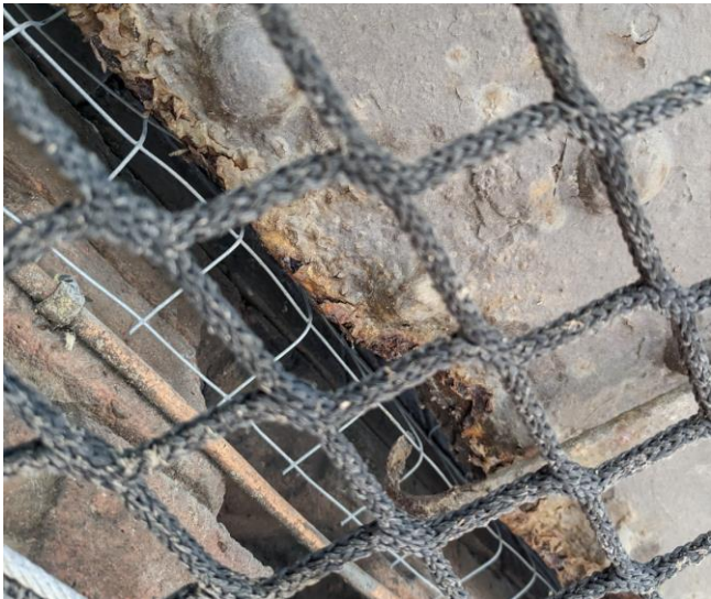
Figure 2-32 Severe corrosion & loss of section width – southern face of south Gantry beam, bottom flange
