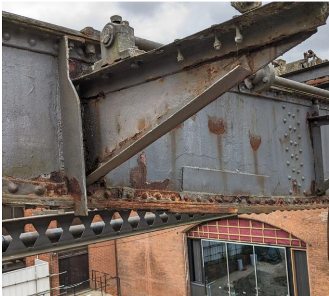
Figure 2-26 Corrosion to bottom of crane beam
