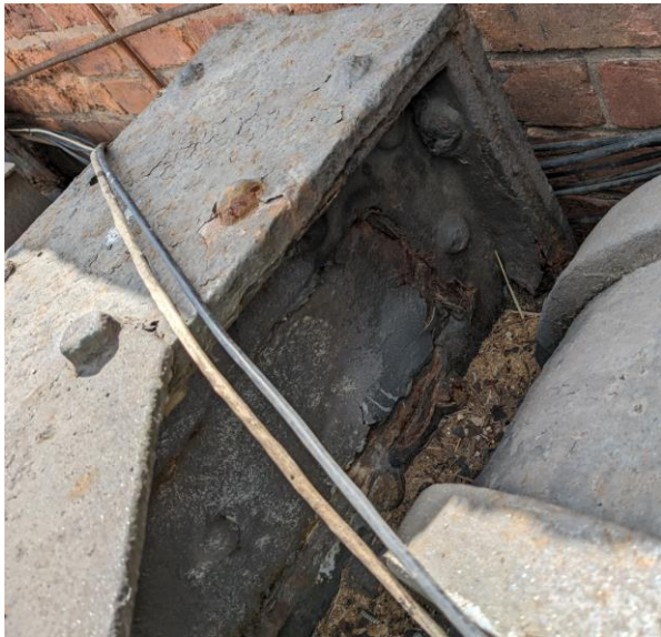
Figure 2-27 Crane beam end corrosion
