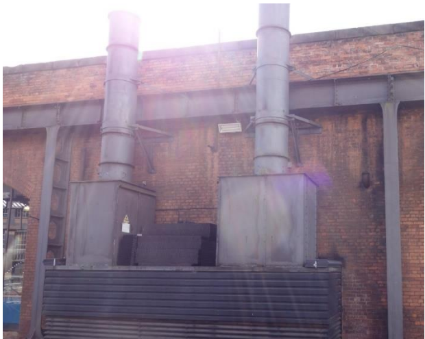
Figure 2-19 – Power Hall chimneys
