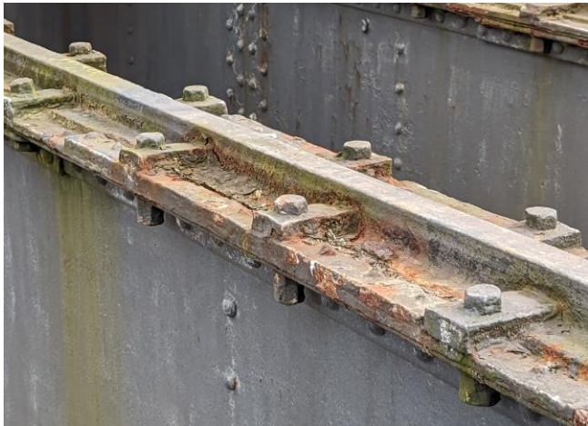
Figure 2-23 Corrosion top face crane beam
