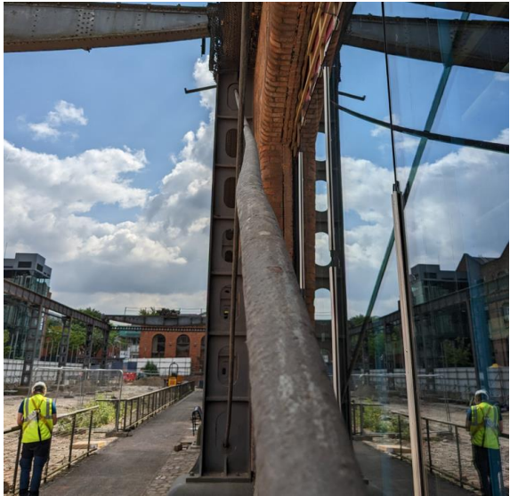
Figure 2-18 South cross bracing showing pitting & deformation
