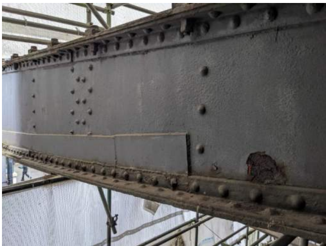
Figure 3-3 Typical example of previous repair
