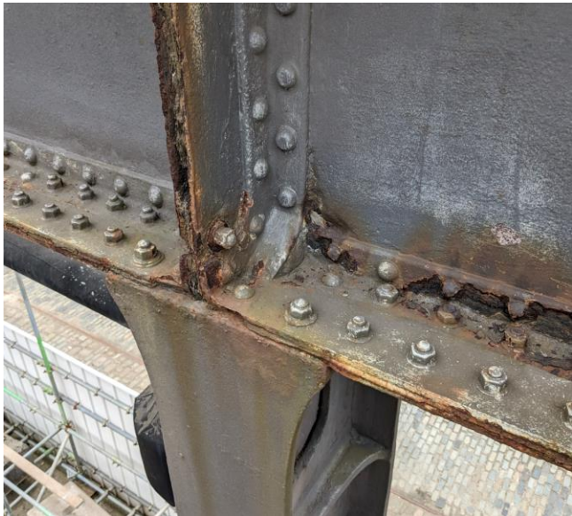
Figure 2-35 Typical corrosion to Gantry beam at column head
