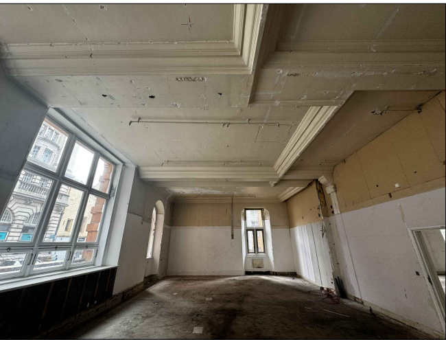
Existing Sprinkler Installation
