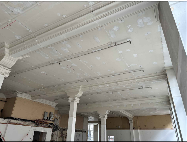
Existing Sprinkler Installation
