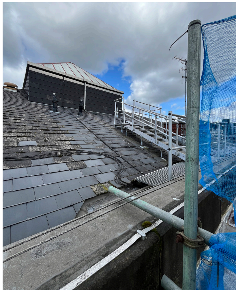
Image 14: Contemporary photograph showing composite tiles and poor condition of roof.
