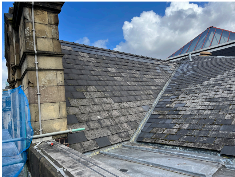
VALLEY AND FLAT ROOF SECTION SHOWING FALLEN TILES
