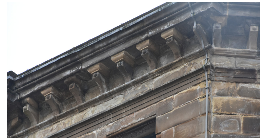
WATER DAMAGE TO PROJECTING STONE
