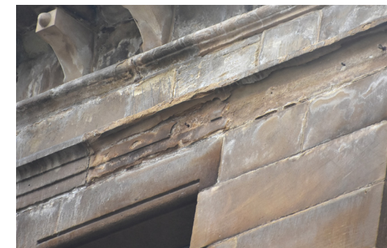
AREAS OF DELAMINATION
