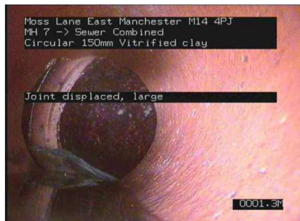
MH 7X_666e0cc9-3183-4dc5-92a9-7255e744a067_20220722_10 3639_165.jpg, 00:00:23, 1.30 m Joint displaced, large
