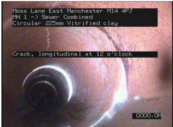
MH 1X_a2d6b3c0-f1c0-44f4-bc3d-94a5009270e1_20220722_134 746_265.jpg, 00:00:16, 0.00 m Crack, longitudinal at 12 o'clock
