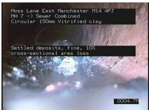
MH 7X_a7565f7d-30c4-4f7e-8027-ba760a1e0e91_20220722_103 715_033.jpg, 00:00:53, 4.70 m Settled deposits, fine, 10% cross-sectional area loss
