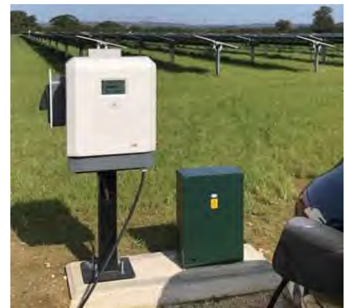
Figure 2 – An R460 Pillar in use for car charging in a GRIDSERVE solar farm
