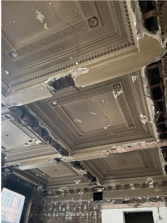
Figure 18: Deteriorated condition of the moulded, coffered plaster ceiling in the former banking hall at ground floor.
