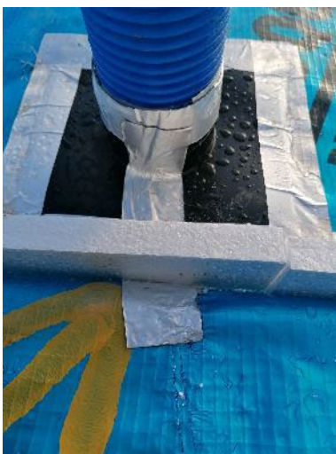
Figure 5 – Gaps in service entries have been correctly sealed.
