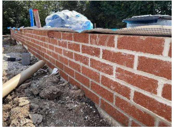
Figure 2 – Sufficient vents can be seen (every 2m).
