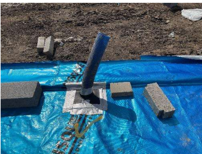
Figure 5 – Service entries patched correctly.
