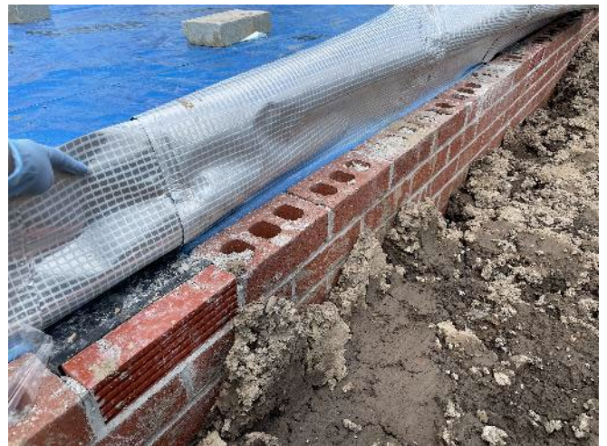
Figure 2 – Sufficient vents can be seen (every 2m).
