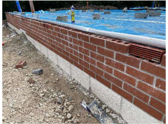
Figure 2 – Sufficient vents can be seen (every 2m).
