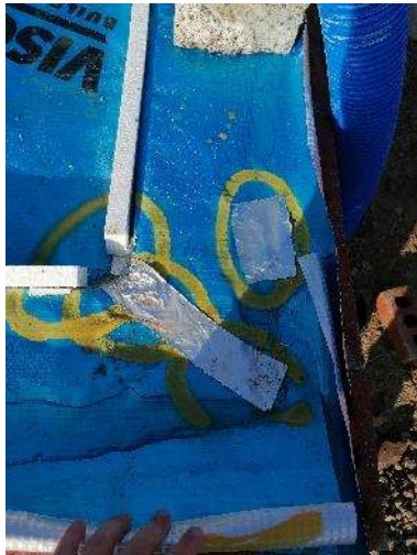
Figure 3 – Gaps in corners correctly sealed.
