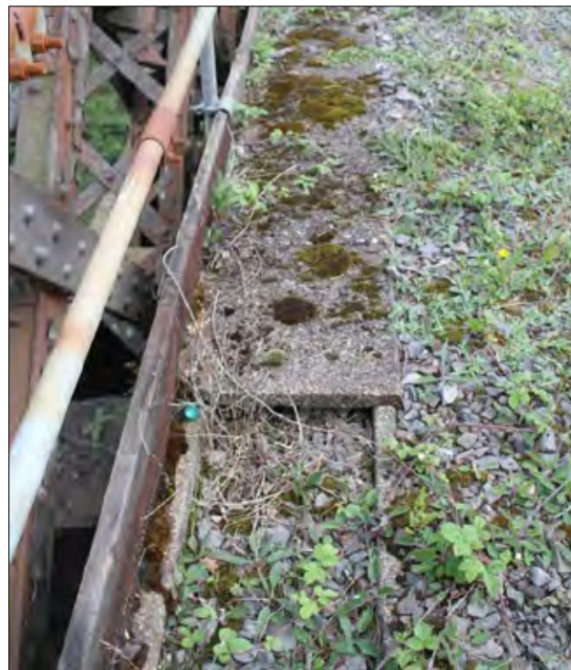
Concrete ducting for electric cabling
