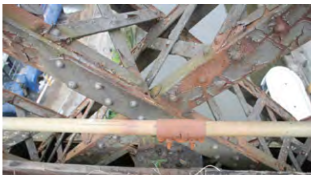
Steel fishplate with angled head showing thinner section and less corroded rivets
