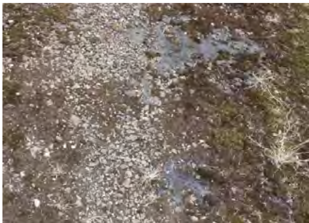
Exposed bitumen on the deck
