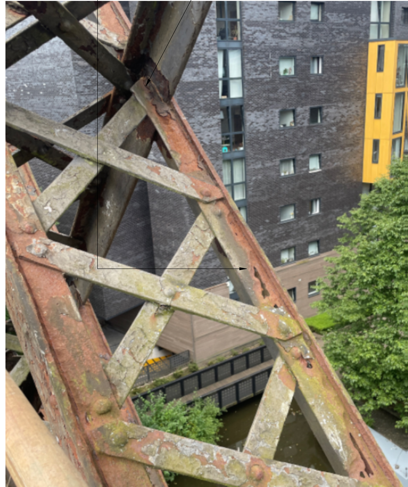
Example 2 - loss of section to outer angle in this example, across 2 bays of X-bracing - at least 2 holes per length of outstand
