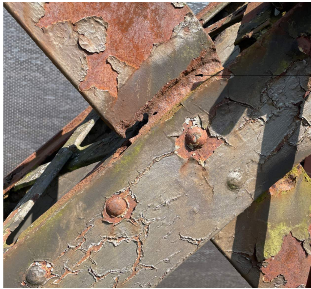
Example 3 - loss of section across less than 50% length of angle web - pitting and loss of thickness elsewhere
