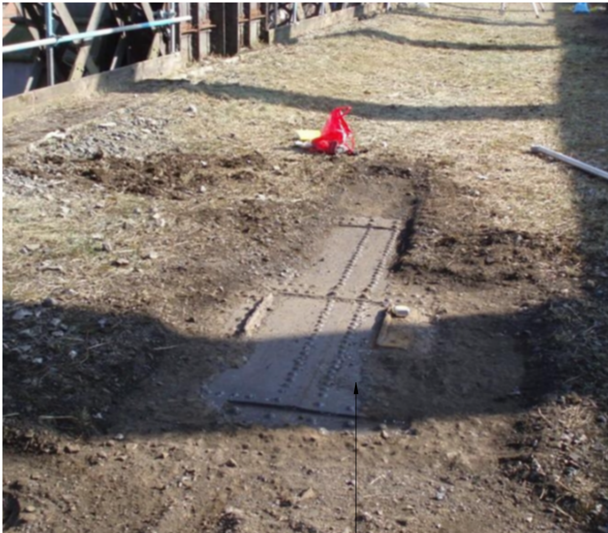
Exposed deck plate and rivets - from Balfour 2020 survey - location unknown - waterproofing not visible
