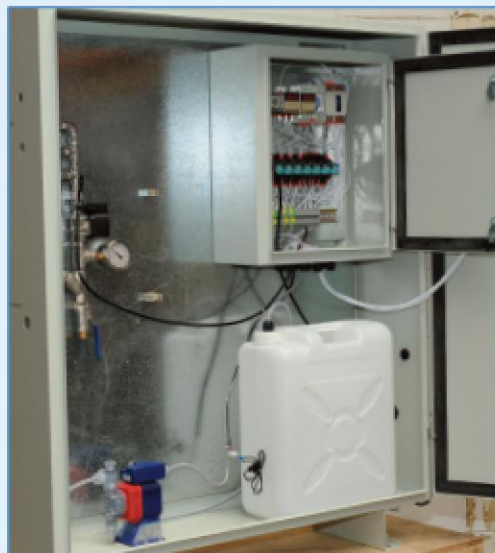
INTERIOR OF AUTOWASH CABINET
