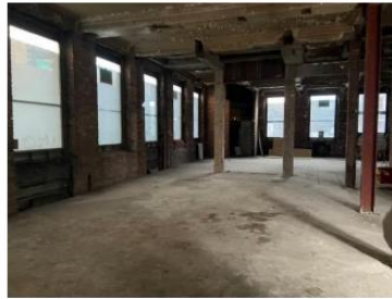
Figure 19: Loss of original partitions at ground floor level has created a large open space, connecting former banking hall with former office spaces.
