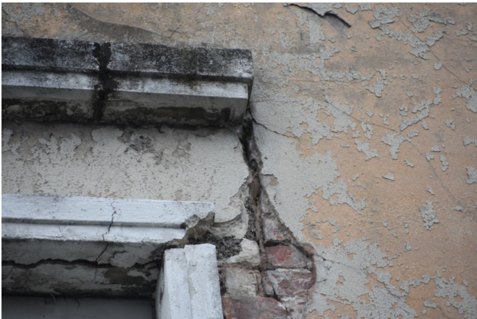
Damaged window head and outer lintel, damaged and missing render
