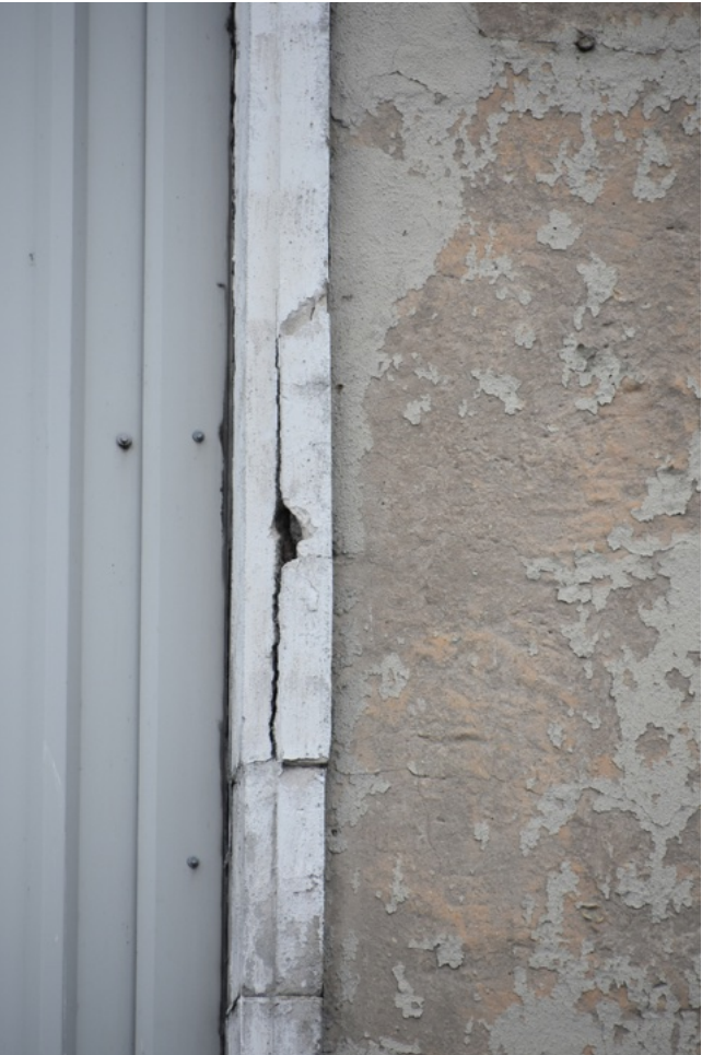
Damaged cast stone to window jamb
