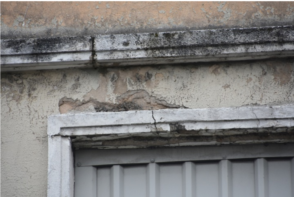
Damaged window head and render, missing grout at cornice
