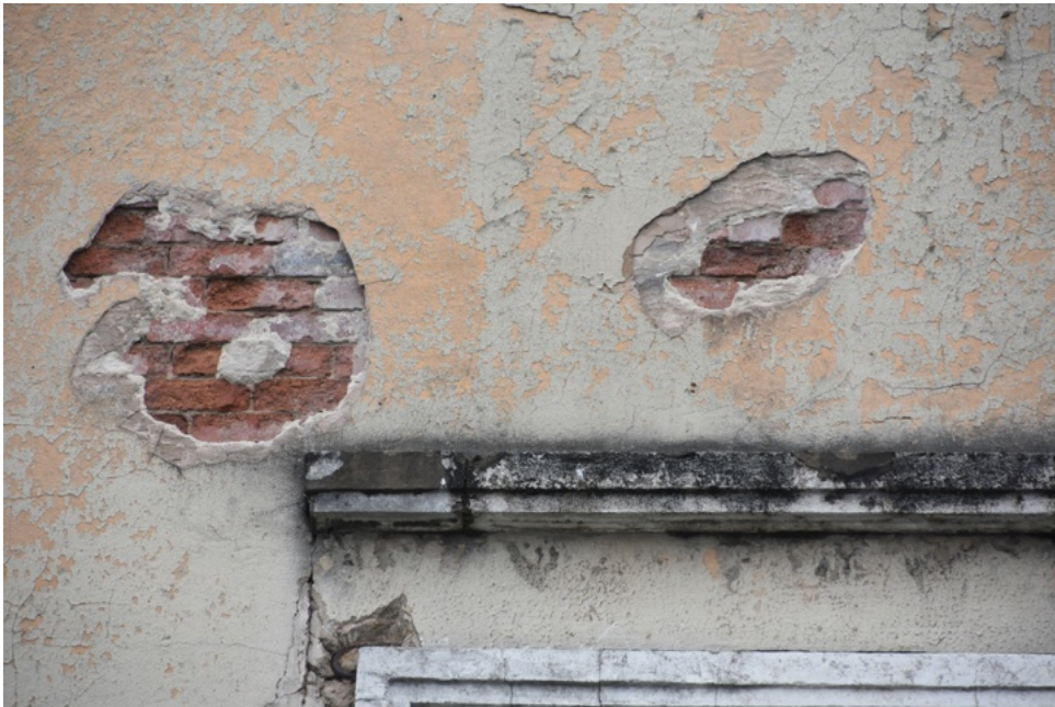
Damaged window head with exposed rebar and missing render
