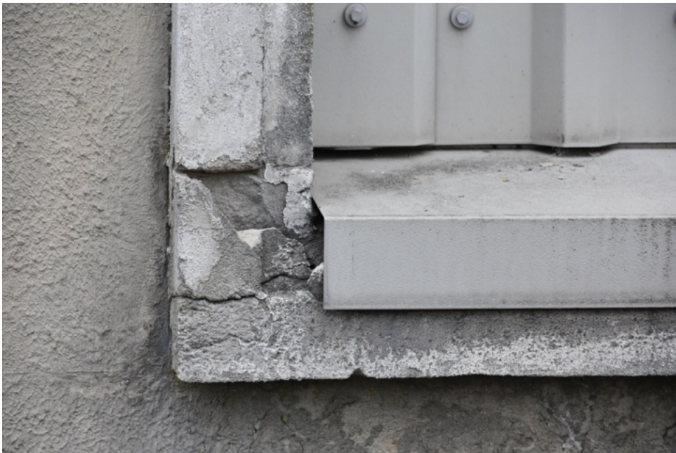
Typical frost damaged cast stone to window surround
