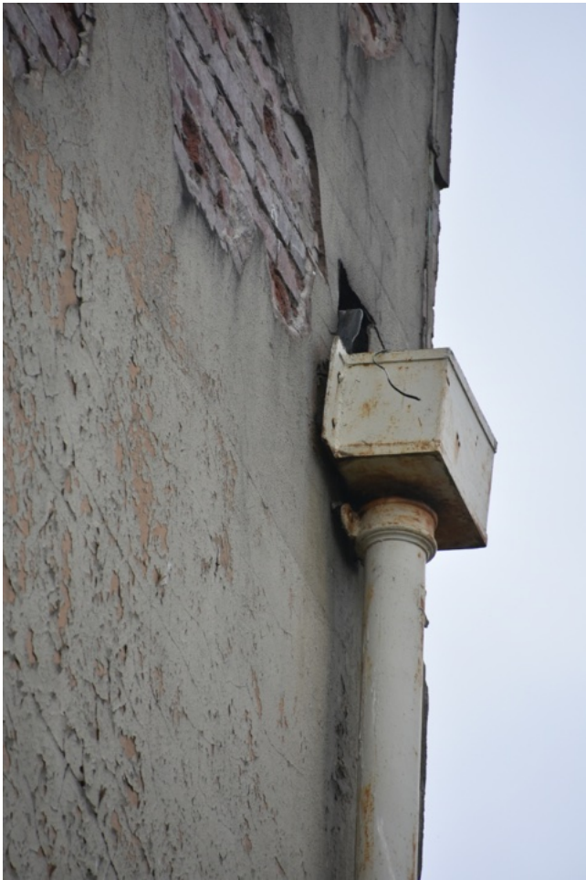
Damaged render and hopper not fixed to wall
