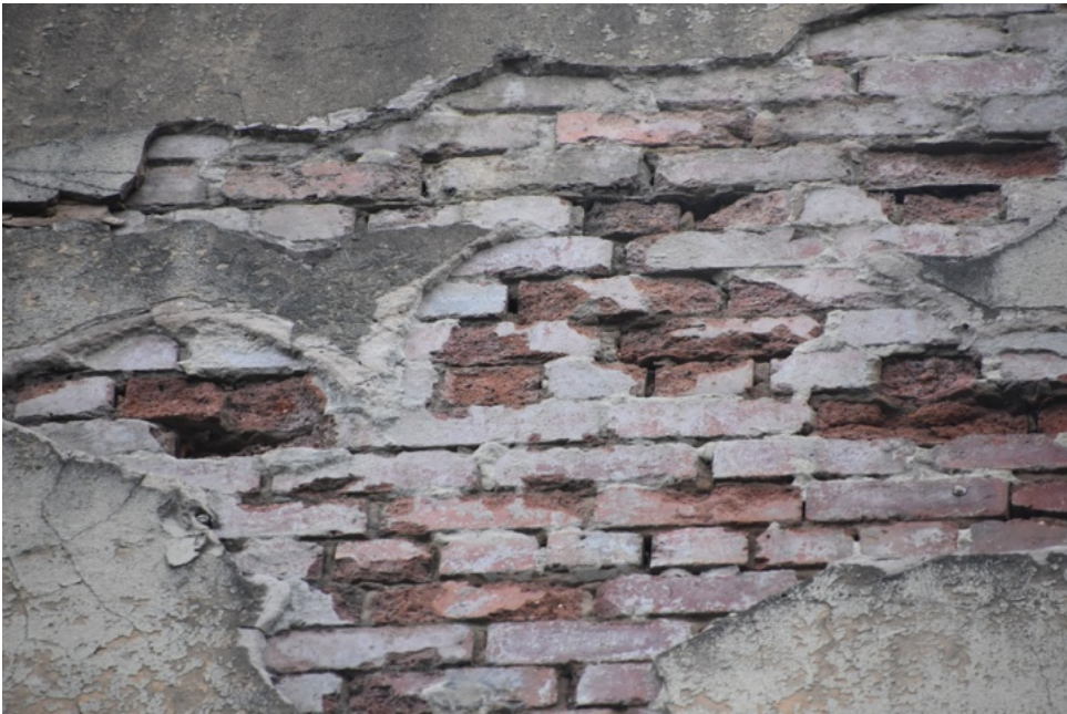
Missing render and frost damaged brickwork
