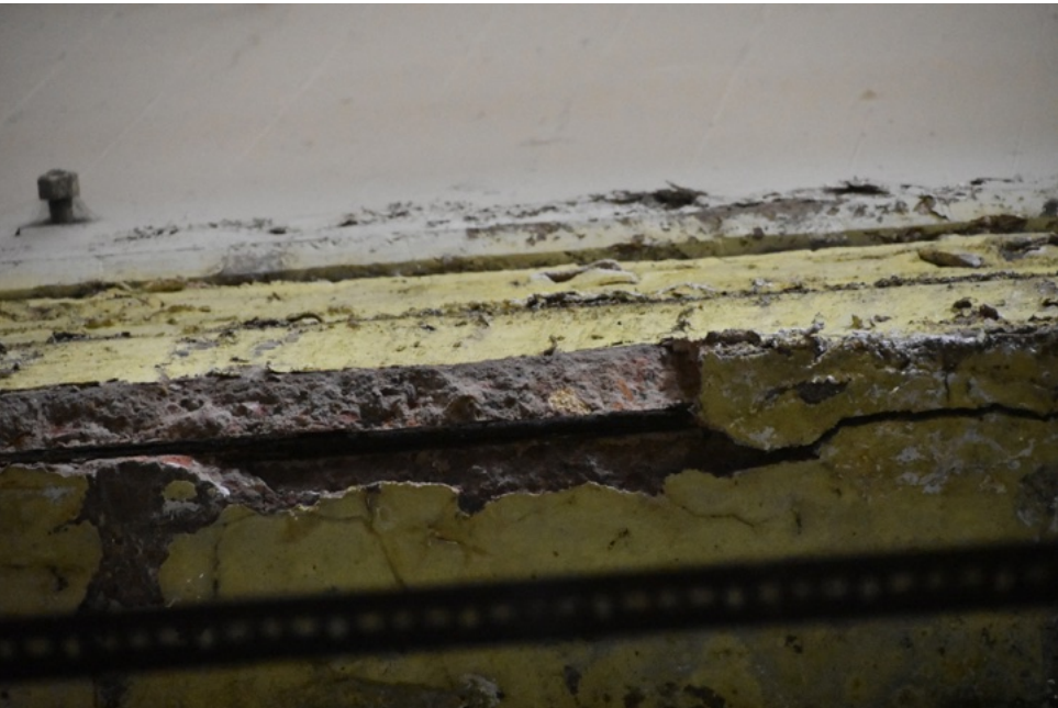
Cracked internal lintel with exposed rebar
