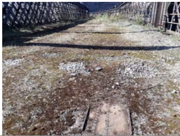
Plate 15: Surface of the viaduct with areas of metal plates visible in parts.
