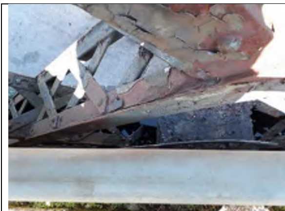
Plate 17: Water collected in part of the viaduct structure on northern side of structure.
