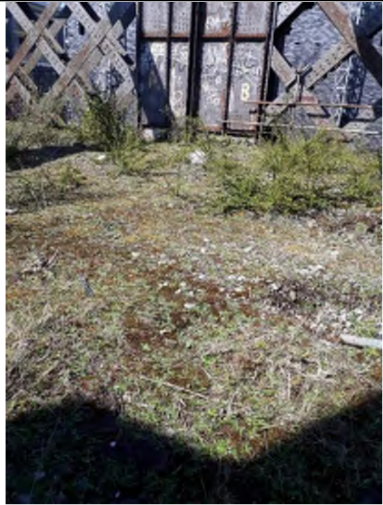
Plate 14: Metal and paint fragments visible on the surface of the viaduct which appear to have originated from the overhead beams.
