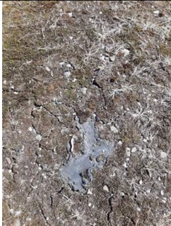
Plate 13: Moss, grasses and plants cover the surface of the viaduct with some small areas of possible tar/bitumen visible.
