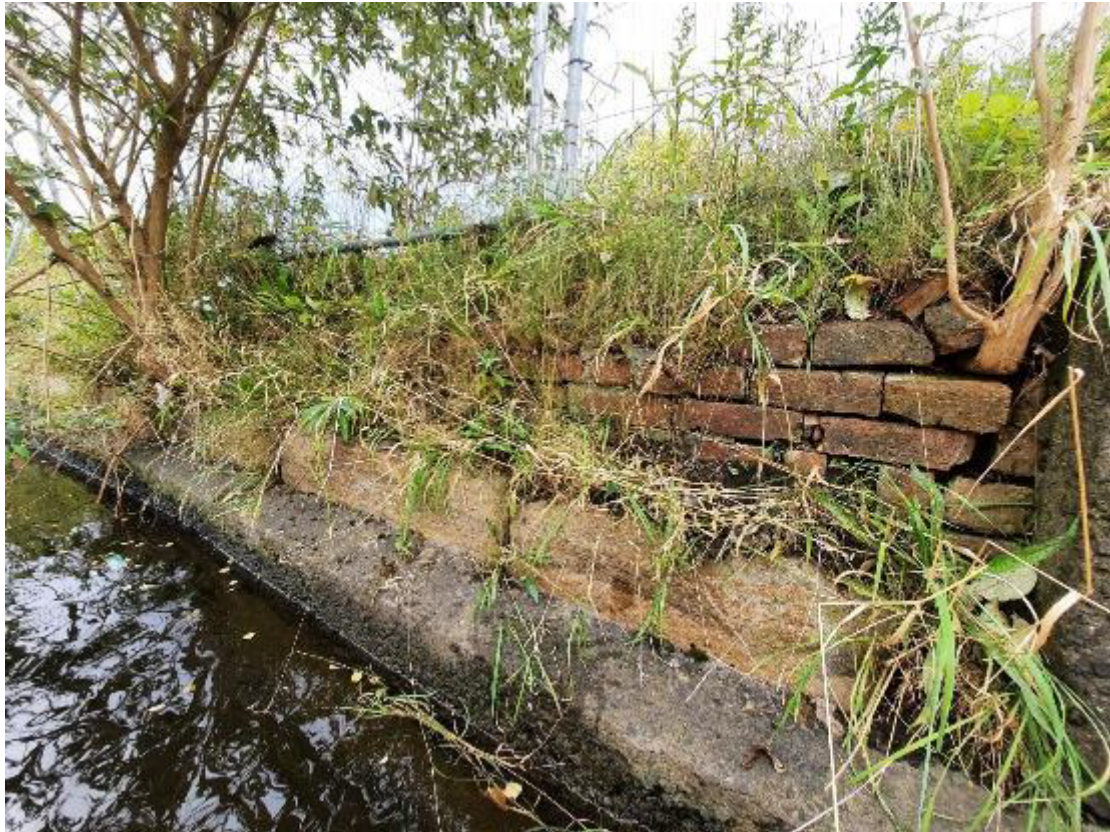
Photo 34: Typical example of joint mortar loss and displacement to brickwork between ch.115m and ch.117m (defect no.23).
