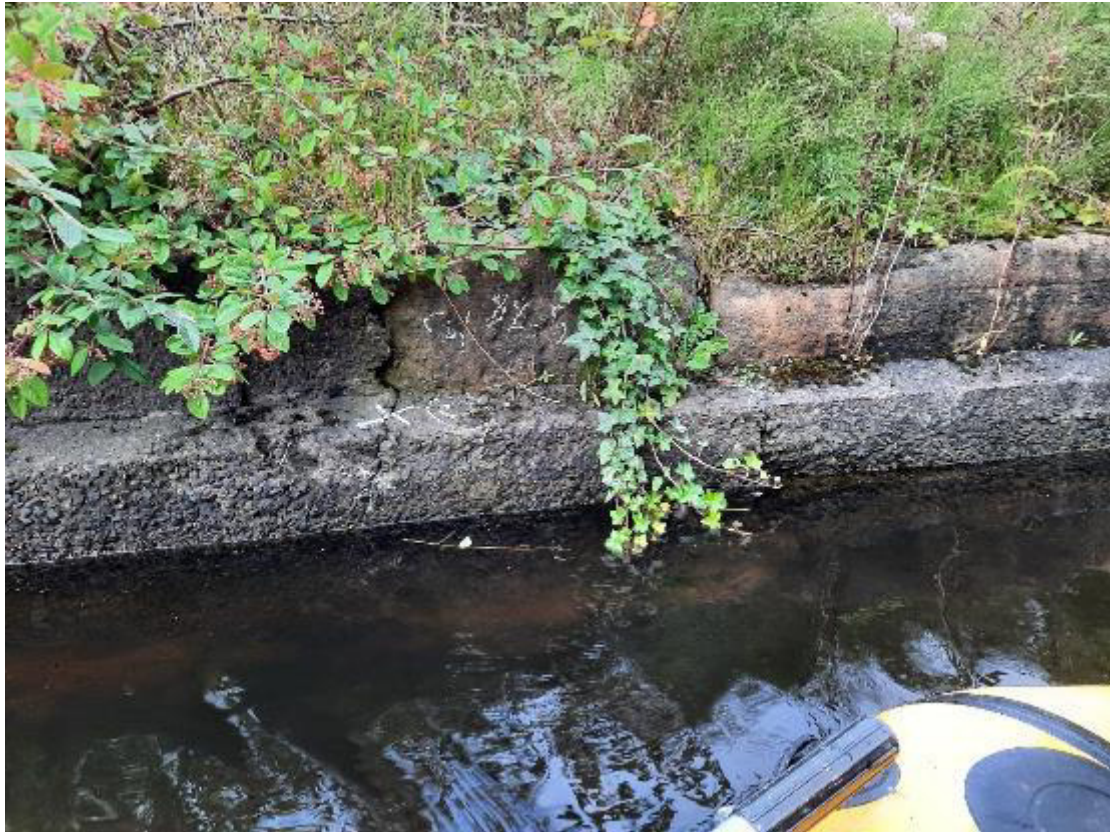
Photo 31: 2 no. vertical cracks to concrete plinth at ch.88.5m (defect no.21).
