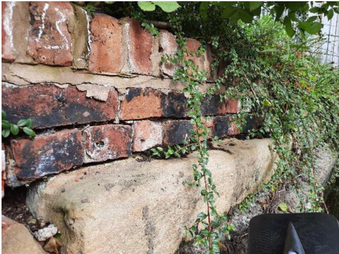
Photo 23: Typical example of joint mortar loss to brickwork between ch.50m & ch.100m (defect no.13).
