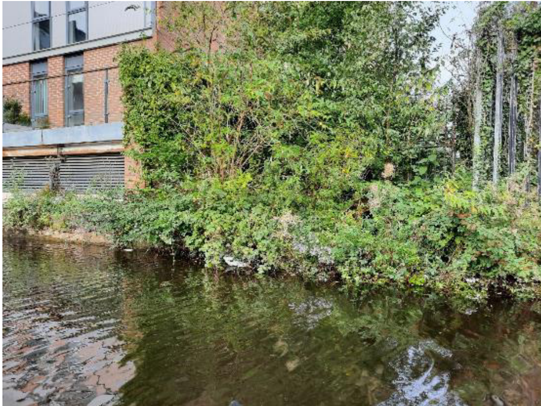
Photo 11: Overgrown vegetation covering wall and affecting full inspection at ch.0.7m (defect no.1)
