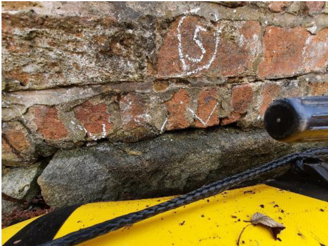
Photo 15: Typical example of joint mortar loss to brickwork between ch.0m & ch.20m (defect no.5).
