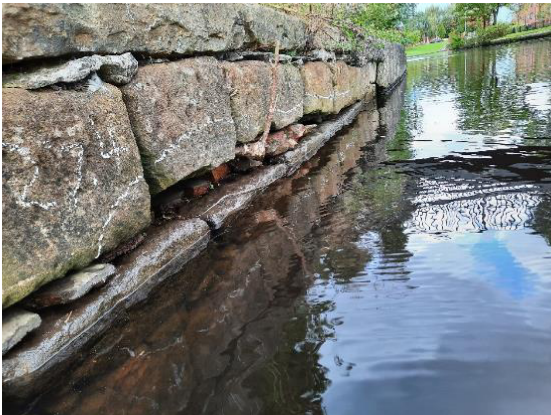
Photo 45: Missing section of stonework at ch.227.5m (defect no.34).
