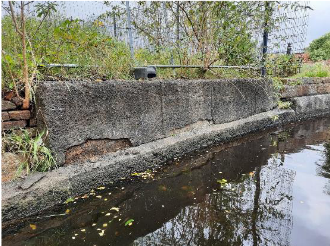
Photo 35: 2 no. areas of spalling to concrete skim over existing stonework at ch.118.6m (defect no.24).
