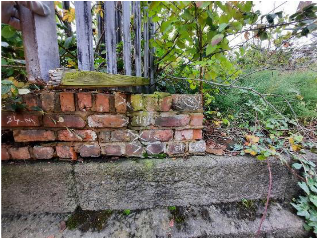
Photo 29: Vertical stepped crack to brickwork at ch.84.7m (defect no.19).
