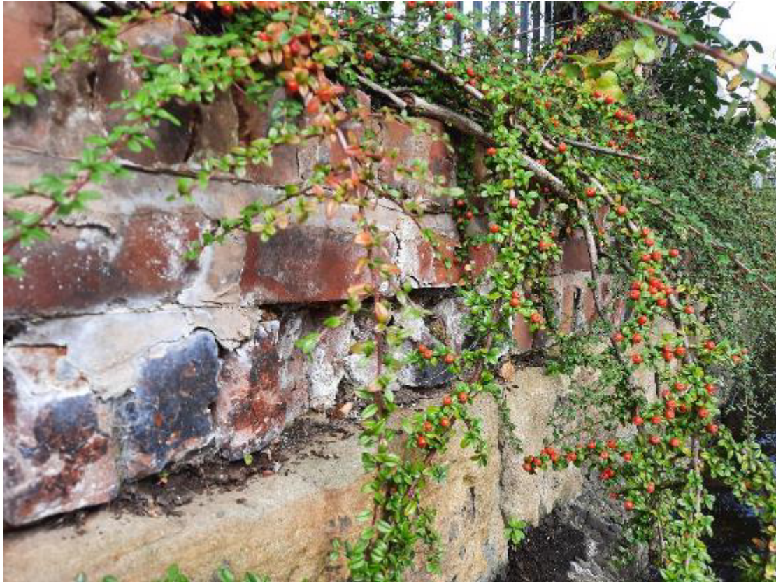
Photo 25: Area of face loss to brickwork at ch.61m (defect no.15).
