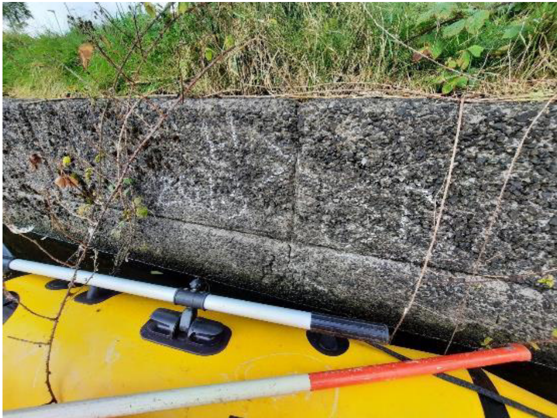
Photo 42: Vertical crack to concrete at ch.207.3m (defect no.31).
