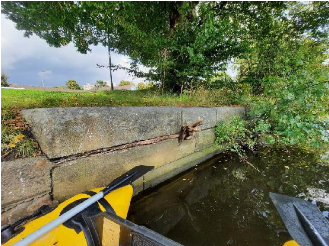
Photo 38: Displaced stonework and associated root growth at ch.145.1m (defect no.27).
