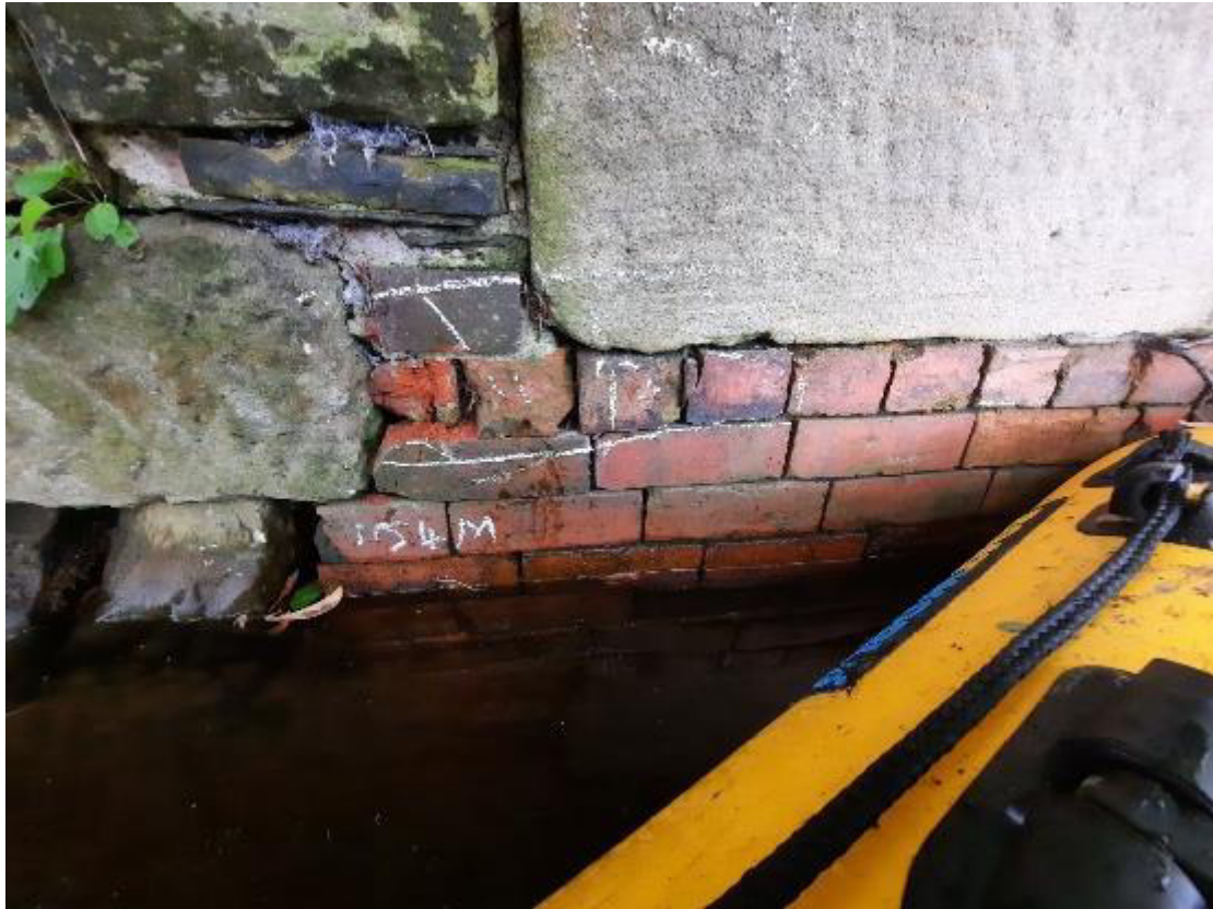
Photo 40: Area of spalled and loose brickwork at ch.154m (defect no.29).
