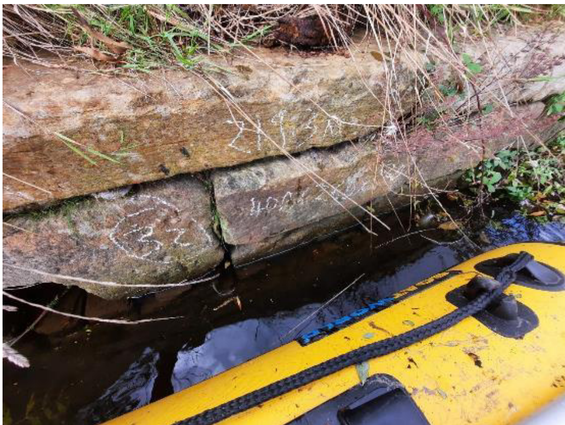
Photo 43: Area of missing stonework below water level at ch.219.5m (defect no.32).
