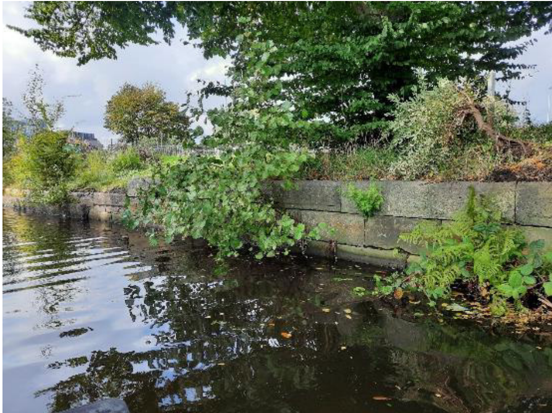
Photo 39: 4 no. areas of sapling growth through stonework between ch.148.5m and ch.160m (defect no.28).
