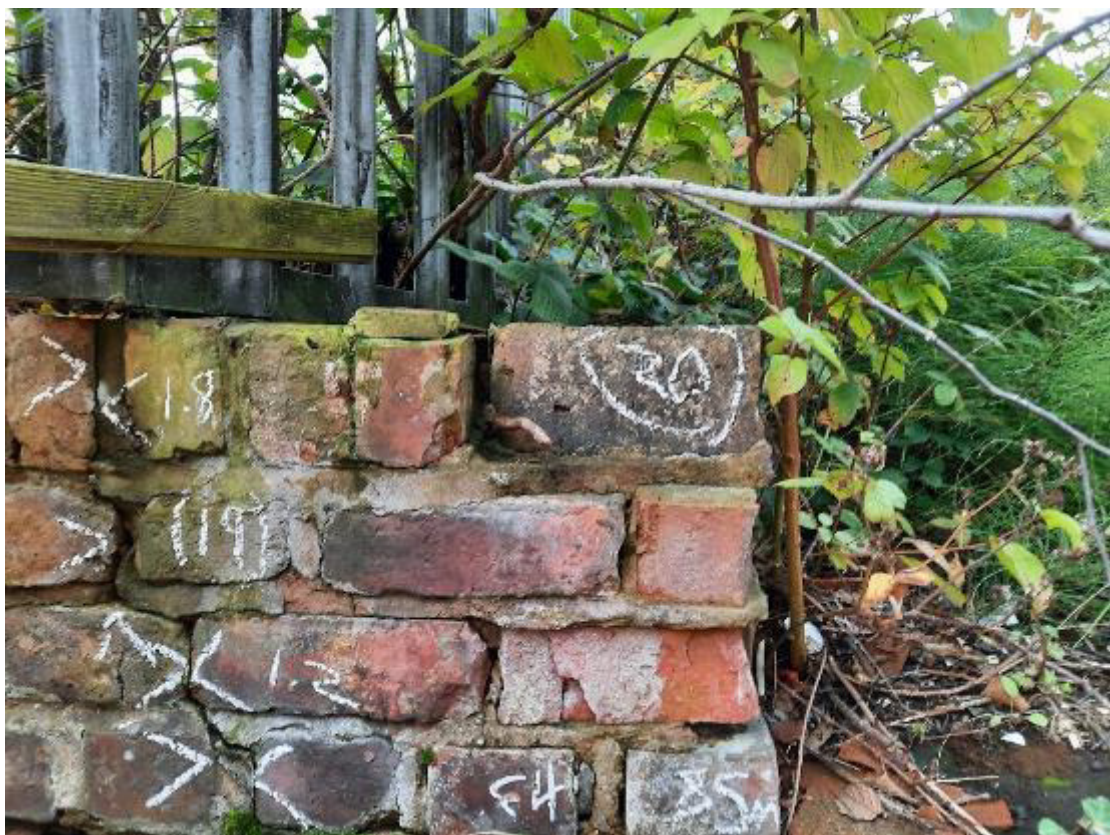
Photo 30: Missing brickwork at ch.85m (defect no.20).
