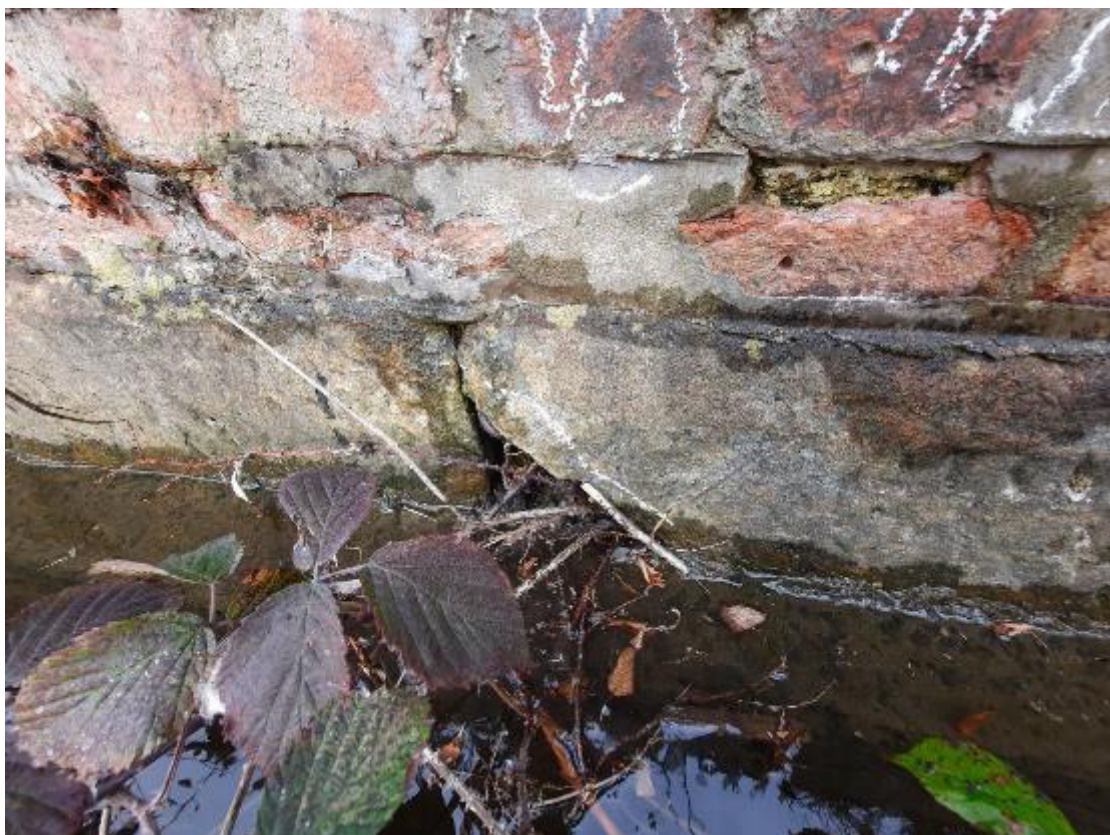
Photo 14: Spall to stonework at ch.15m (defect no.4).
