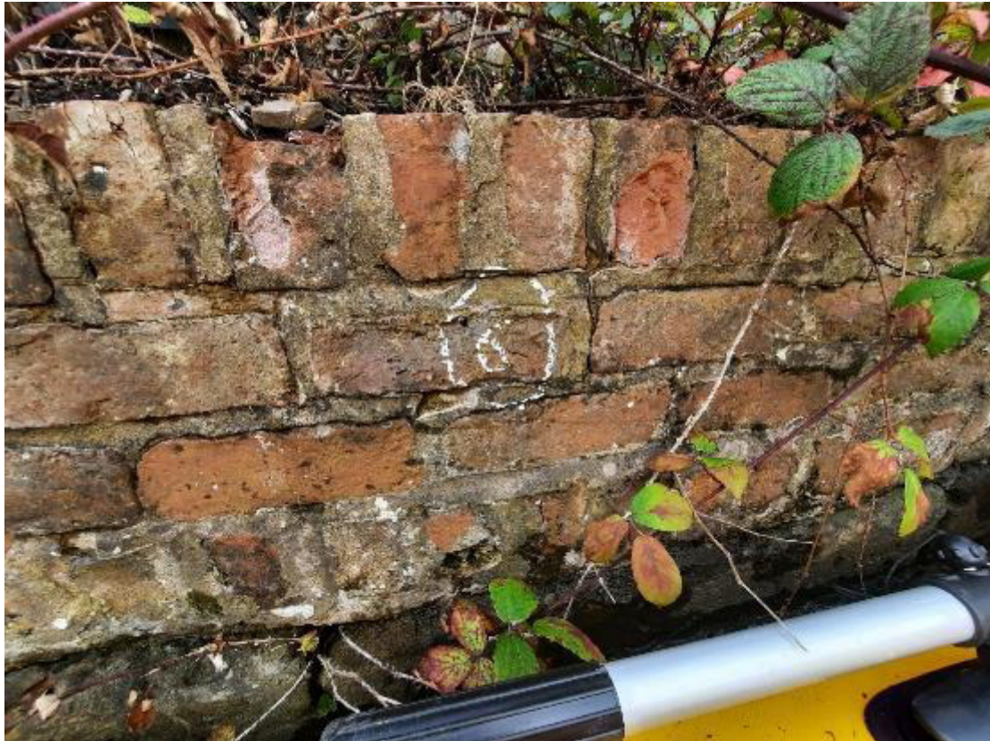
Photo 16: Typical example of face loss to brickwork between ch.0m and ch.20m (defect no.6).
