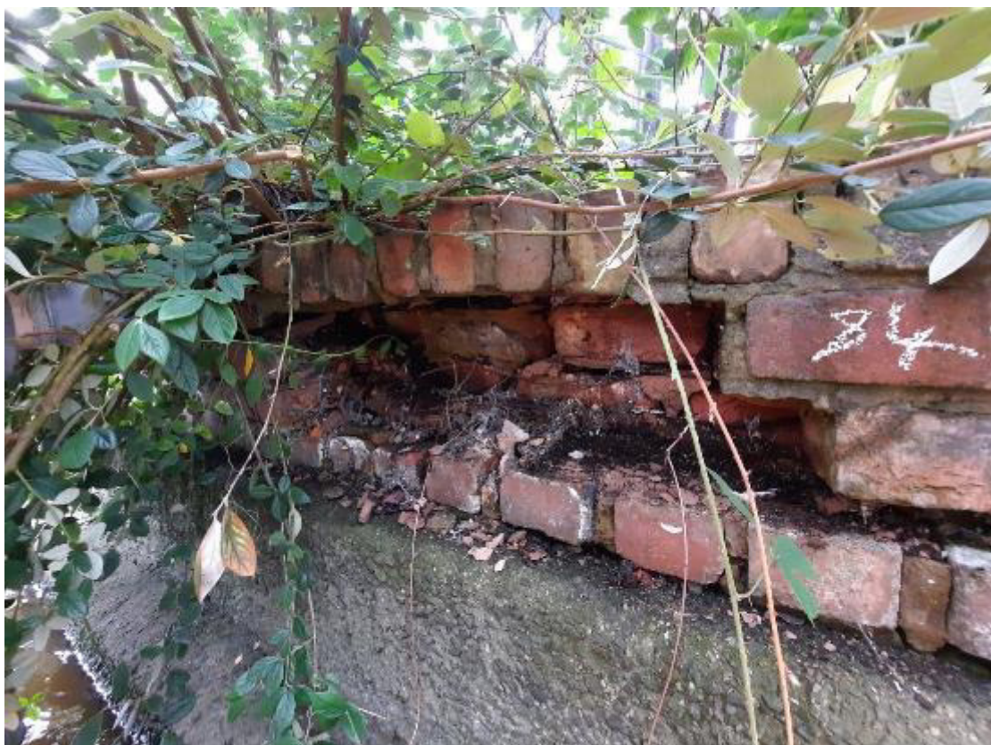
Photo 28: Missing section of brickwork at ch.84m (defect no.18).
