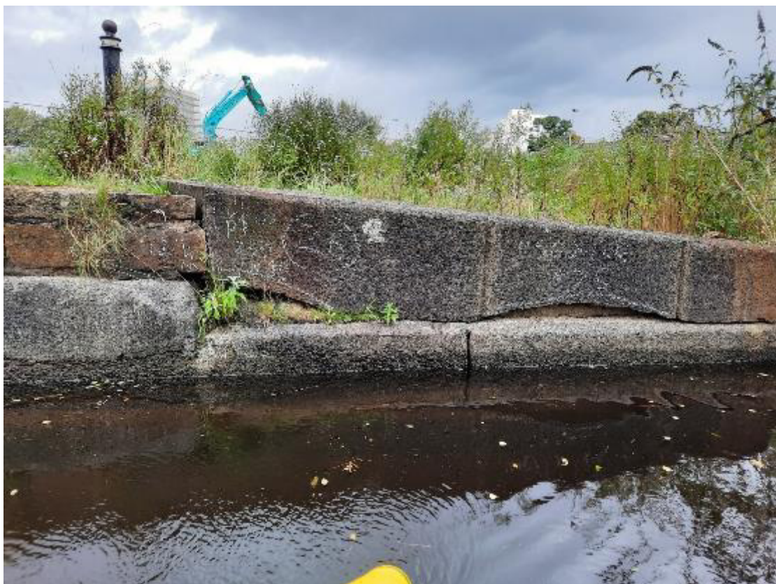
Photo 37: 2 areas of spalled concrete at ch.124m (defect no.26).
