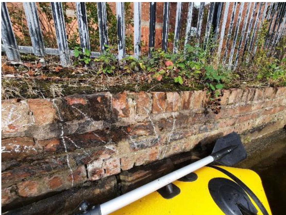
Photo 18: Area of hollow sounding and loose brickwork at ch.22m (defect no.8).
