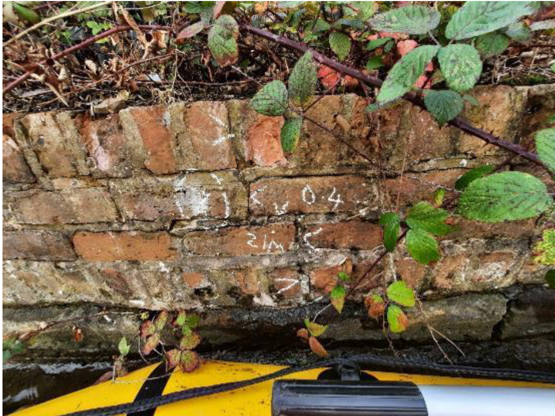
Photo 17: Vertical stepped crack to brickwork at ch.22m (defect no.7).
