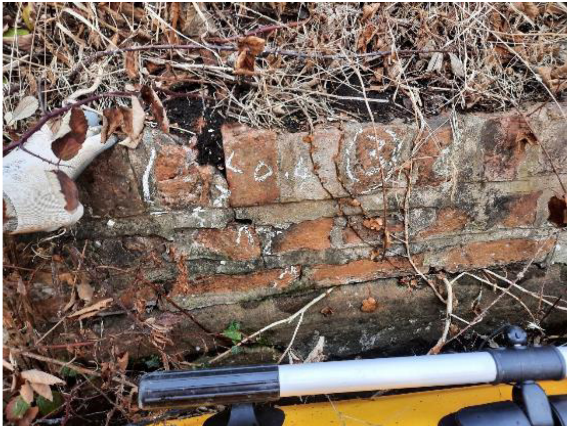
Photo 13: Vertical stepped crack to brickwork at ch.13m (defect no.3).
