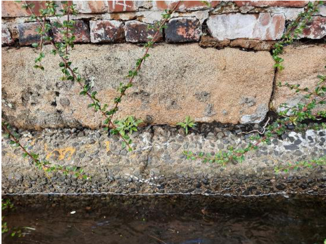
Photo 24: Vertical crack to concrete plinth at ch.56.5m (defect no.14).
