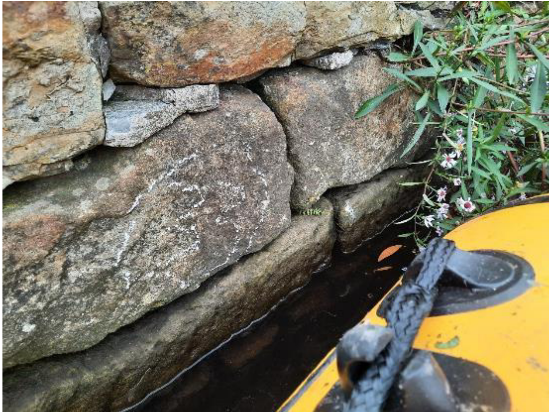
Photo 44: Typical example of joint mortar loss to stonework between ch.219m & ch.230.5m (defect no.33).
