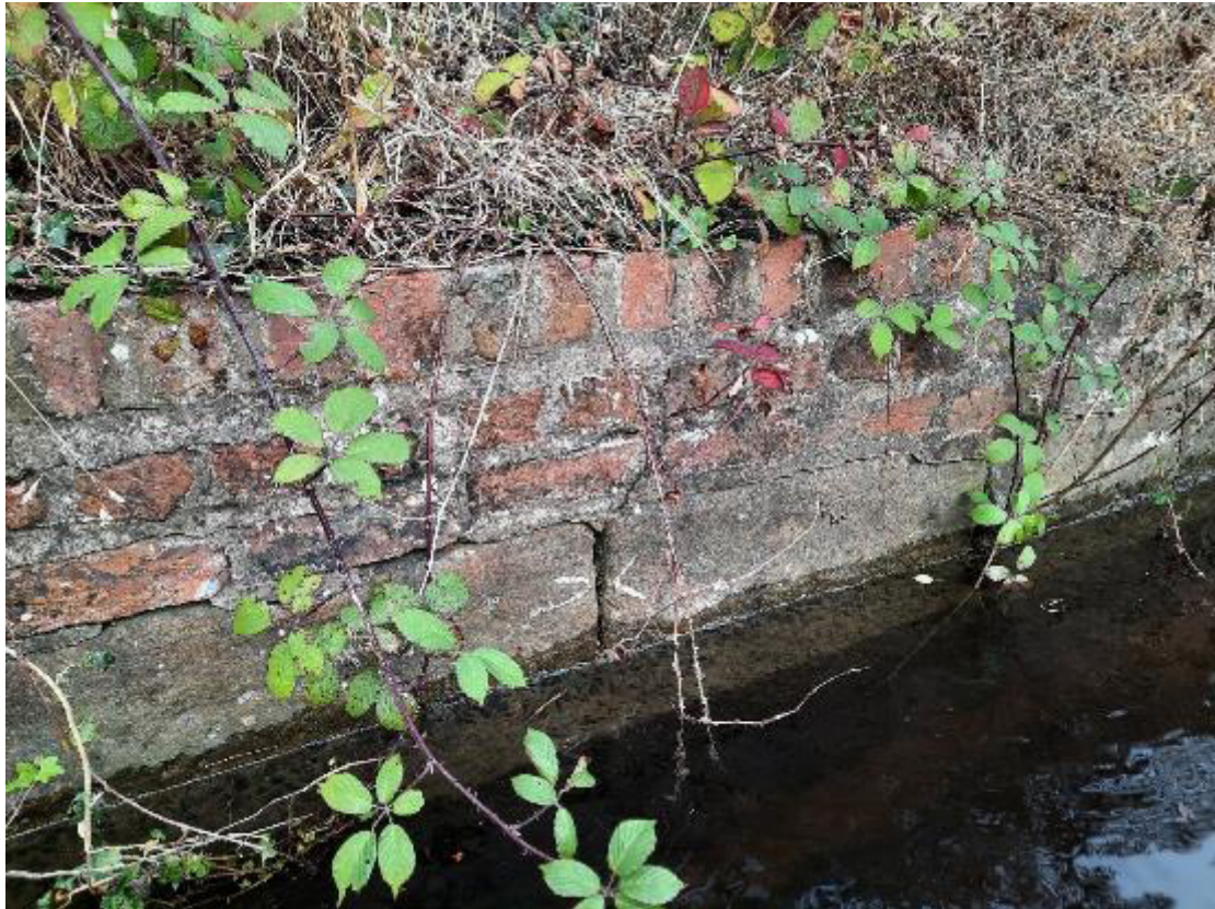
Photo 12: Typical example of joint mortar loss to stonework between ch.10m & ch.50m (defect no.2).
