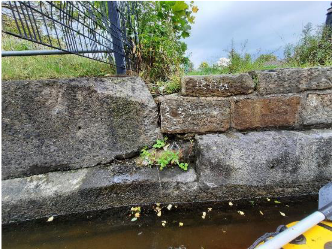
Photo 36: Poor construction joint at ch.120m (defect no.25).
