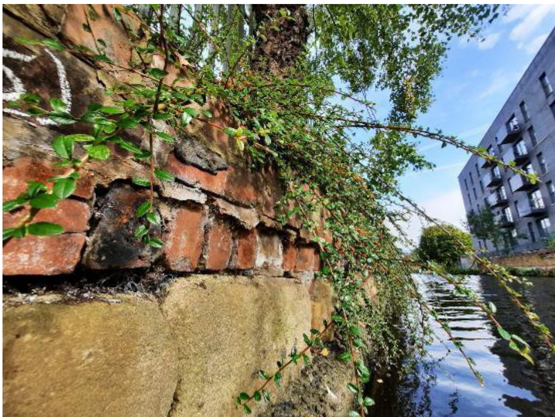
Photo 26: Area of bulged brickwork and associated tree growth from ch.63.6m to ch.65m (defect no.16).
