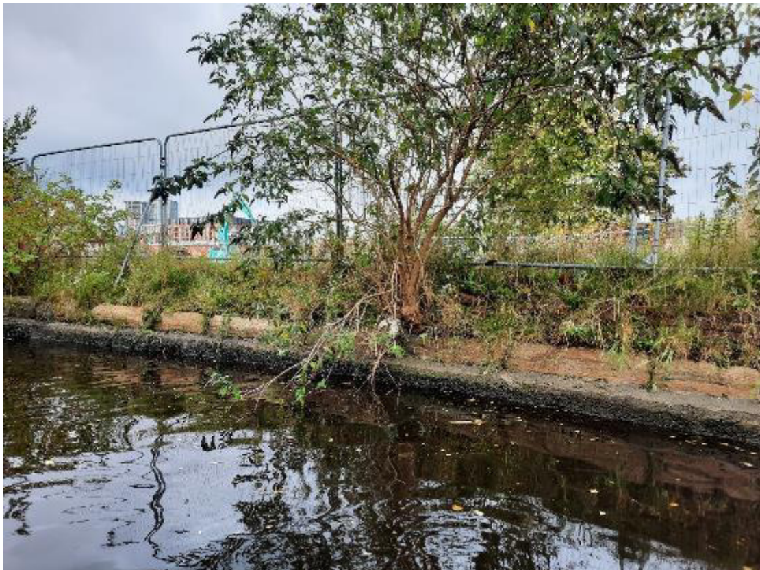
Photo 33: Tree growth adjacent to wall at ch.115m (defect no.22).
