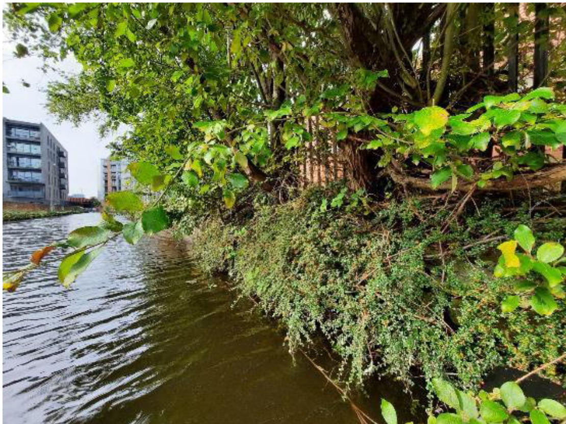
Photo 20: Overgrown vegetation covering wall and affecting full inspection between ch.20m & ch.36.5m (defect no.10).
