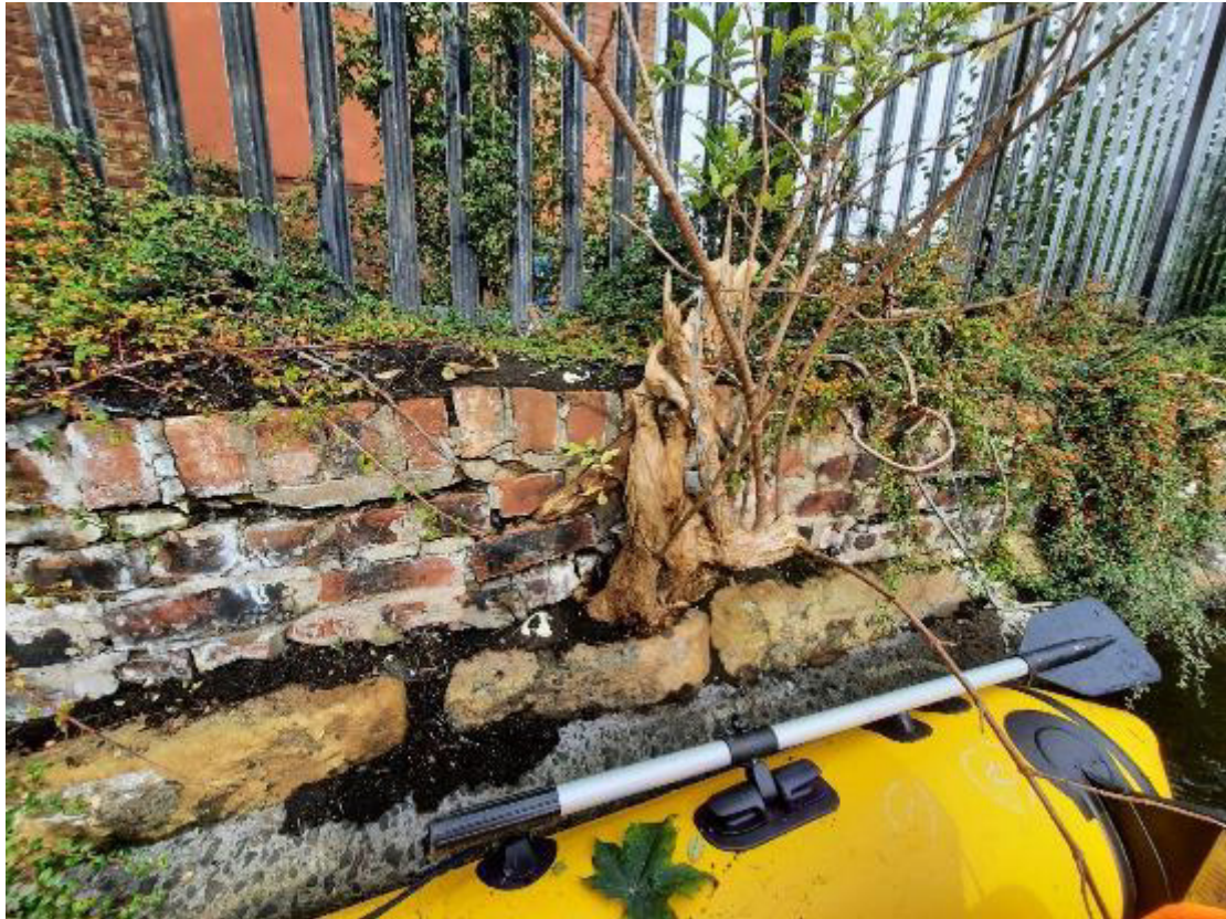
Photo 21: Displaced brickwork and associated root growth from ch.39m to ch.42m (defect no.11).
