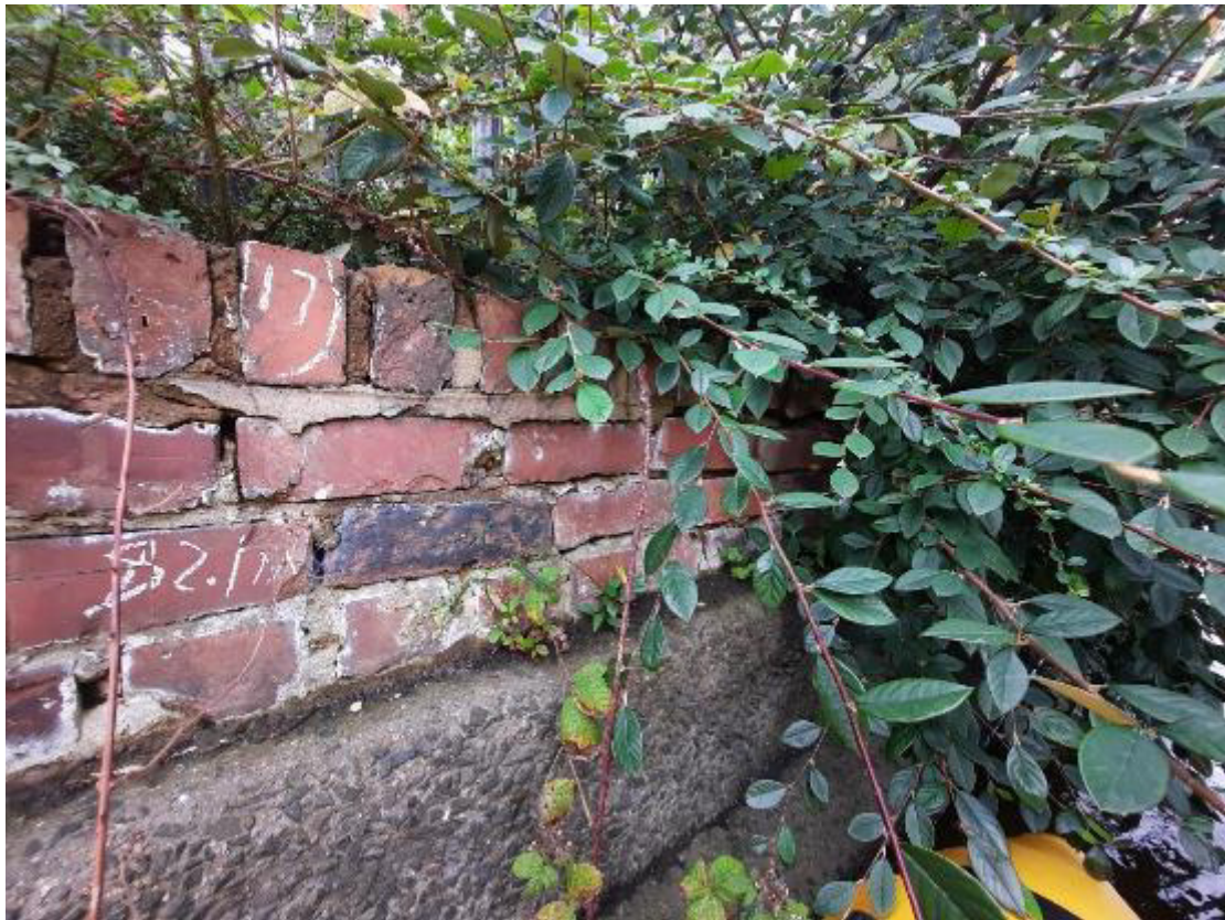
Photo 27: Area of outward displacement to brickwork at ch.82.1m (defect no.17).
