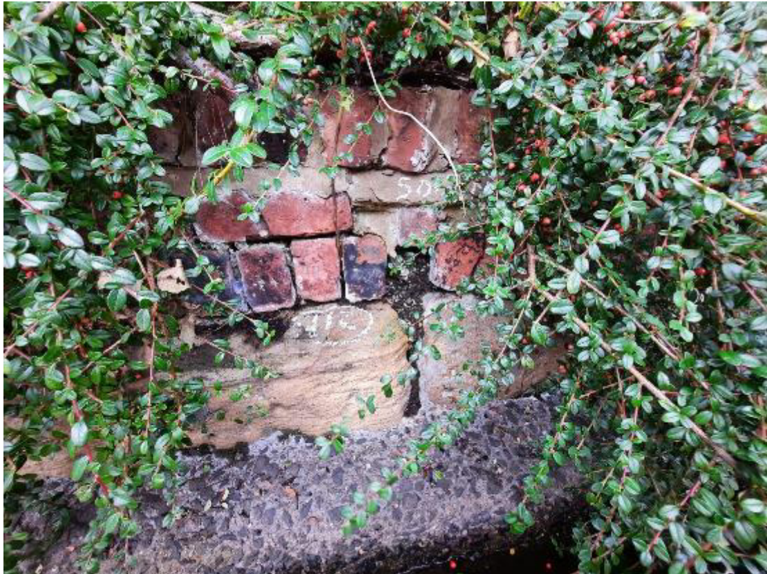
Photo 22: Missing brickwork at ch.50.2m (defect no.12).
