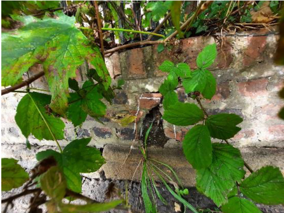
Photo 19: Spall to brickwork at ch.30m (defect no.9).
