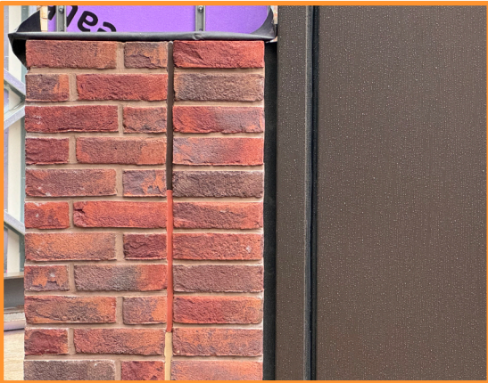
VMU - TOWER INTERFACE
