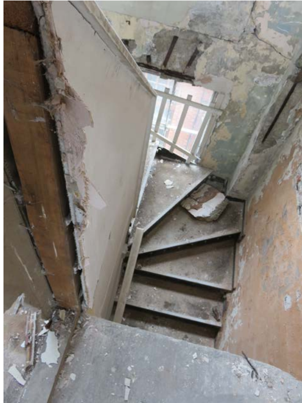
View looking to missing parapet of the stairs on 2 nd Floor.
