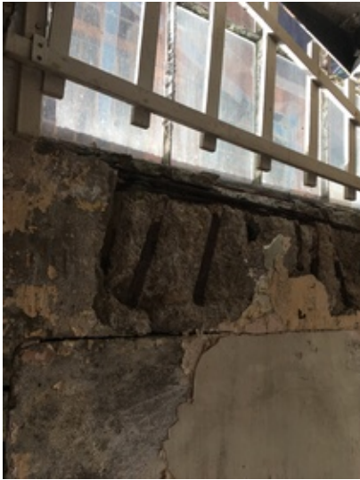
Severe spalling of concrete to the window surrounds with exposed rebar in a number of places.
