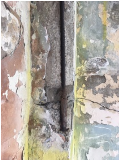
Evidence of spalled concrete and severe cracking to columns with exposed reinforcement.
