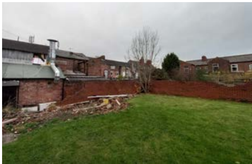
View of the eastern corner of the site showing collapsed boundary wall.
