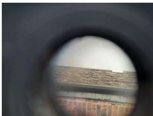
Plate 4.10: Lifted Tiles and Degraded Fascia to the South.
