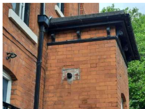
Plate 4.4: Flat Roof Porch Area to East With Some Mortar Degradation in Areas.
