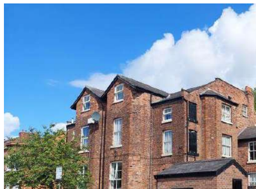
Plate 4.13: South Elevation; Showing Worn Fascia Boards and Broken Windows.
