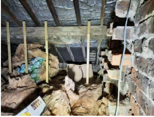
Plate 4.17: Foil Lined Roof Felting Visible to the West
