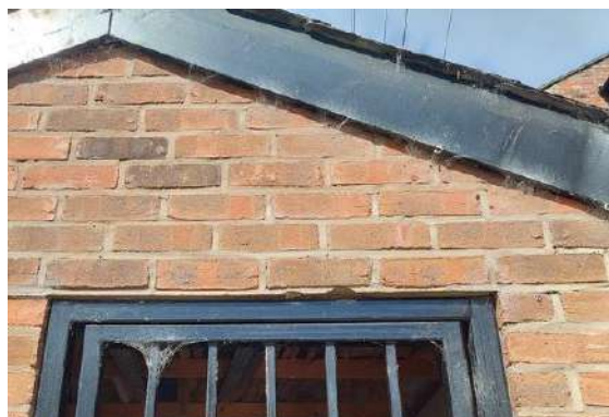
Plate 4.19: Cobwebbing along Fascia Boards
