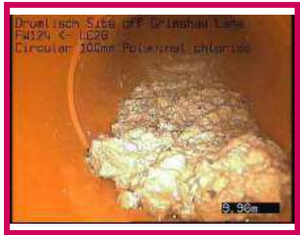
2, 00:00:56, 9.94 m Settled deposits, coarse, 20% cross-sectional area loss
