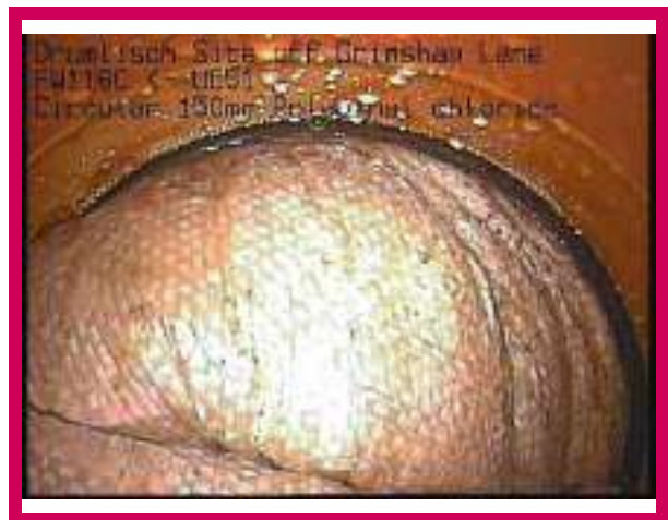
4, 00:01:45, 12.74 m Finish node, other special chamber, reference: UC51, Capped
