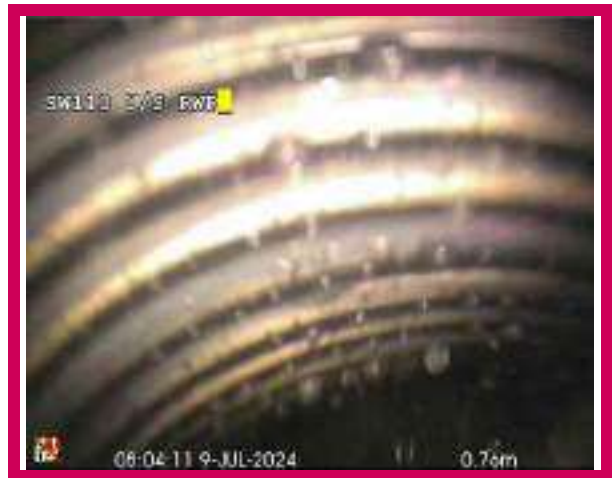
2, 00:00:08, 0.76 m Finish node, other special chamber, reference: RWP, In bottom of RWP
