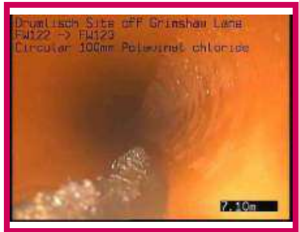
2, 00:00:26, 7.10 m Settled deposits, fine, 5% cross-sectional area loss
