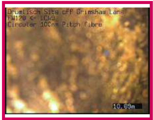
2, 00:00:52, 10.69 m Finish node, gully, reference: UC49
