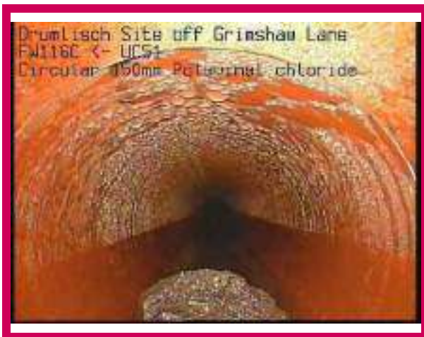
3, 00:00:47, 4.65 m Settled deposits, coarse, 10% cross-sectional area loss
