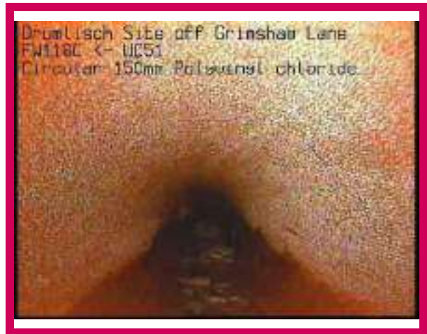
2, 00:00:41, 3.67 m Settled deposits, hard or compacted, 5% cross-sectional area loss
