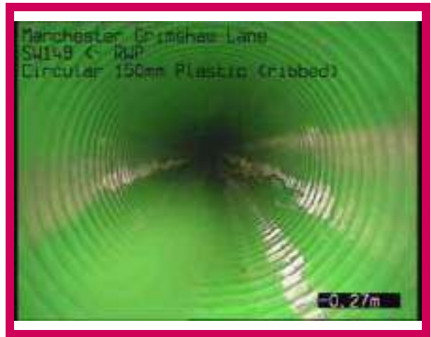
2, 00:01:29, 11.20 m Finish node, other special chamber, reference: RWP, In RWP
