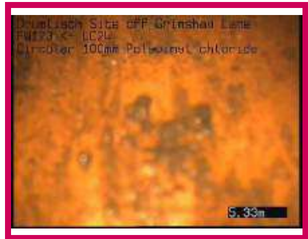
2, 00:00:31, 4.71 m Settled deposits, fine, 5% cross-sectional area loss
