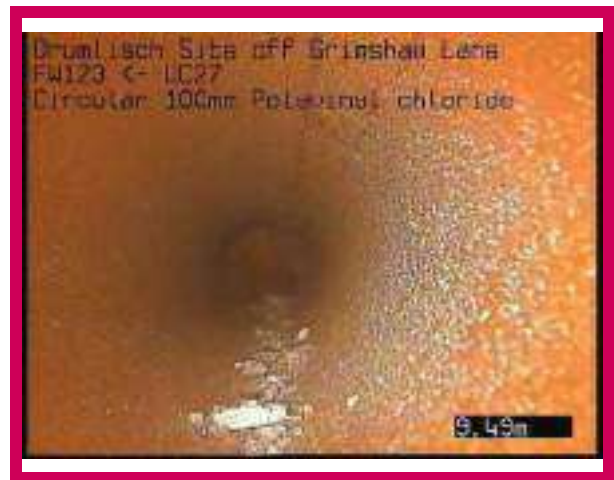
2, 00:00:51, 9.41 m Settled deposits, fine, 5% cross-sectional area loss
