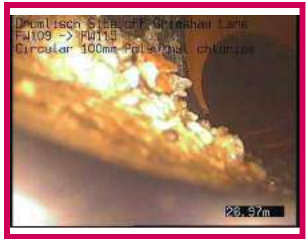
2, 00:01:38, 26.97 m Finish node, manhole, reference: FW115, Main
