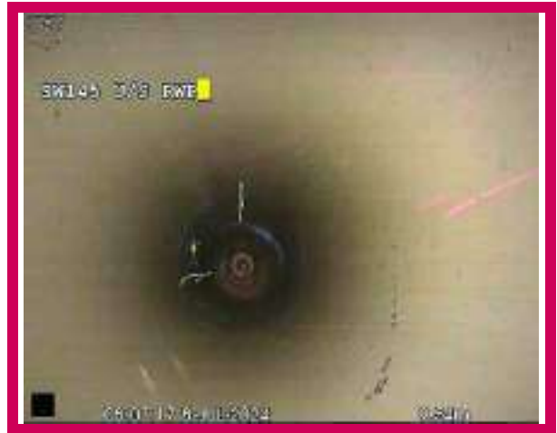
2, 00:00:40, 9.54 m Finish node, other special chamber, reference: RWP, In RWP
