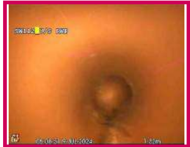
2, 00:00:06, 1.32 m General remark, Material change of pipe. to smooth plastic
