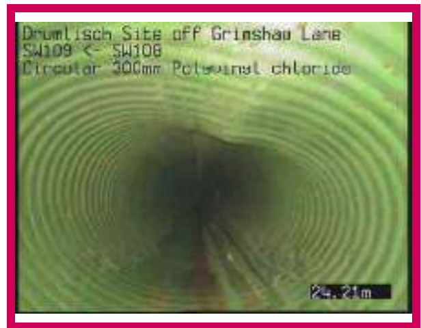
2, 00:02:32, 24.21 m Deformed sewer or drain, 10%
