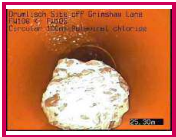
2, 00:02:32, 25.30 m Settled deposits, coarse, 80% cross-sectional area loss
