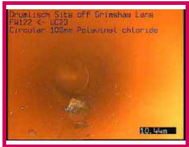
2, 00:01:13, 10.44 m Settled deposits, fine, 5% cross-sectional area loss
