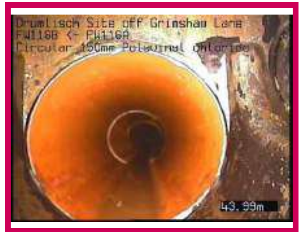
2, 00:04:56, 43.99 m Finish node, manhole, reference: FW116A
