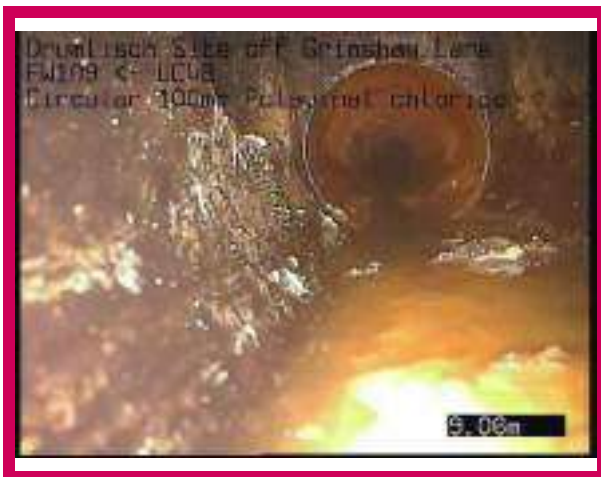
3, 00:00:26, 9.06 m Finish node, manhole, reference: UC48
