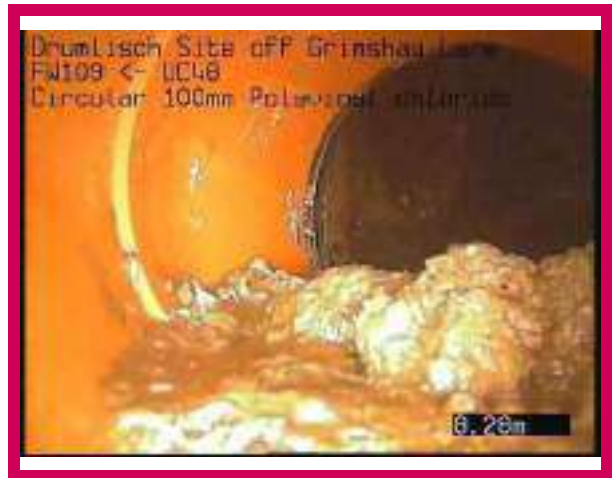
2, 00:00:20, 8.28 m Settled deposits, fine, 20% cross-sectional area loss
