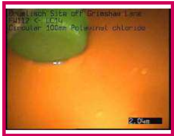
2, 00:00:22, 2.04 m Other obstacles, other object in invert at 6 o'clock, 10% cross-sectional area loss, Bottle in line
