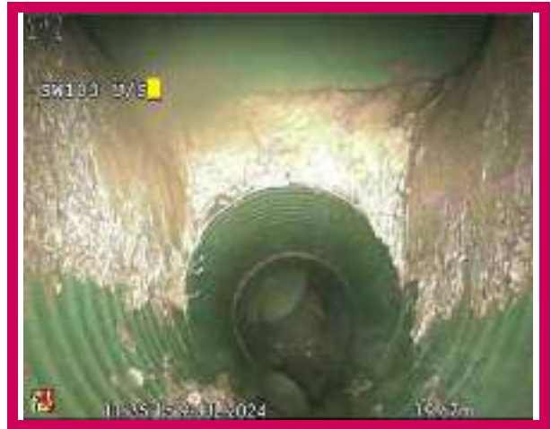
2, 00:01:06, 19.67 m Finish node, manhole, reference: Unmarked, MH not marked on plan.
