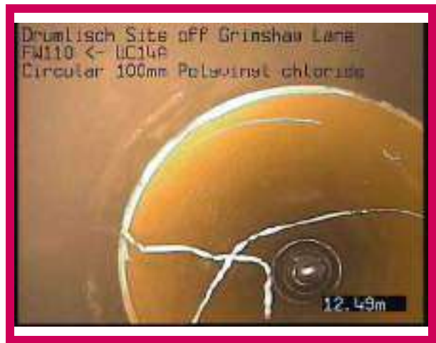
2, 00:01:10, 12.49 m Roots, fine at joint
