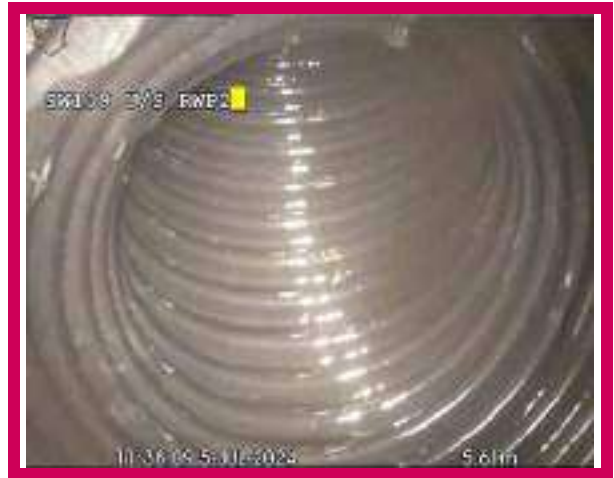
2, 00:00:39, 5.61 m Finish node, other special chamber, reference: RWP2, Pipe material changes back to ribbed plastic and goes up to RWP.
