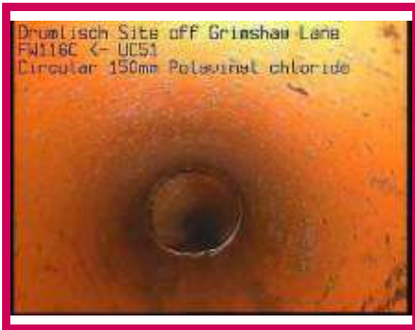
1, 00:00:00, 0.00 m Start node, manhole, reference: FW116C
