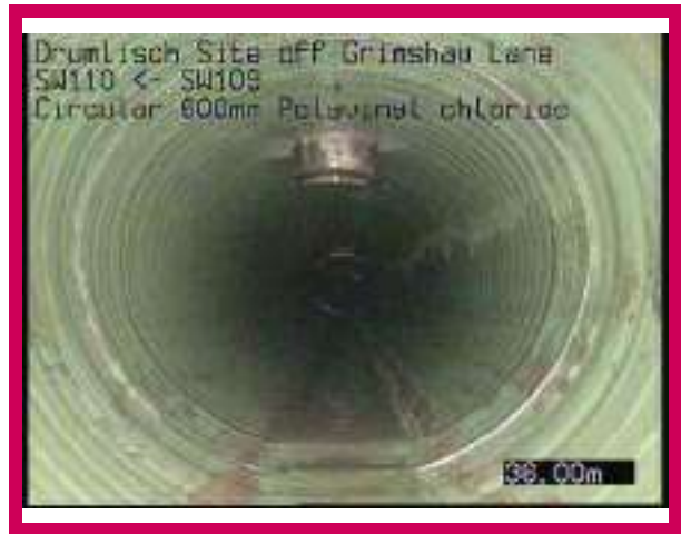
2, 00:02:34, 36.09 m Connection defective, connecting pipe is intruding at 12 o'clock, 150mm dia, intrusion: 5%
