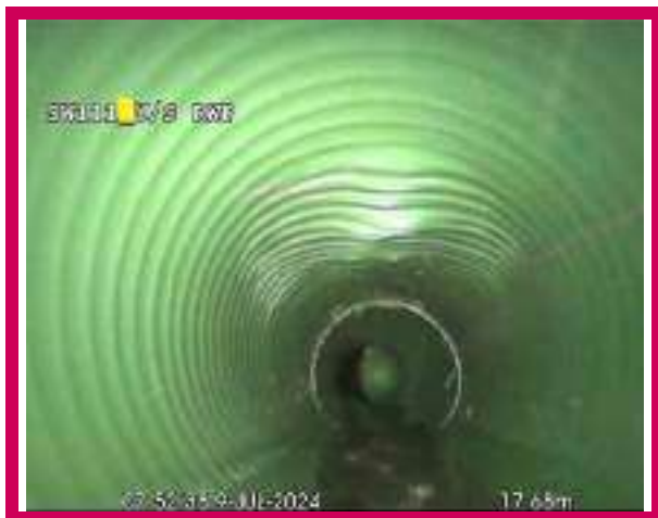
3, 00:00:52, 17.68 m Deformed drain or sewer, 10%
