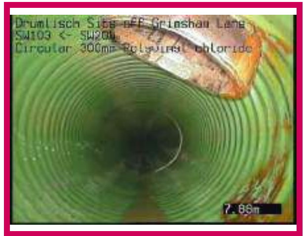
2, 00:00:57, 7.88 m Connection defective, connecting pipe is intruding at 01 o'clock, 150mm dia, intrusion: 10%
