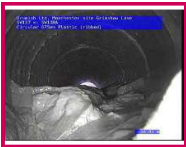
3, 00:02:45, 36.82 m Finish node, manhole, reference: SW138A, Rubble in buried chamber
