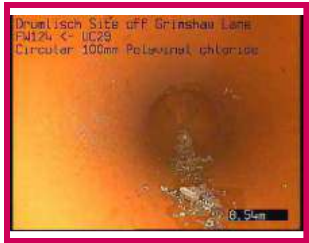
2, 00:00:47, 8.50 m Settled deposits, fine, 5% cross-sectional area loss
