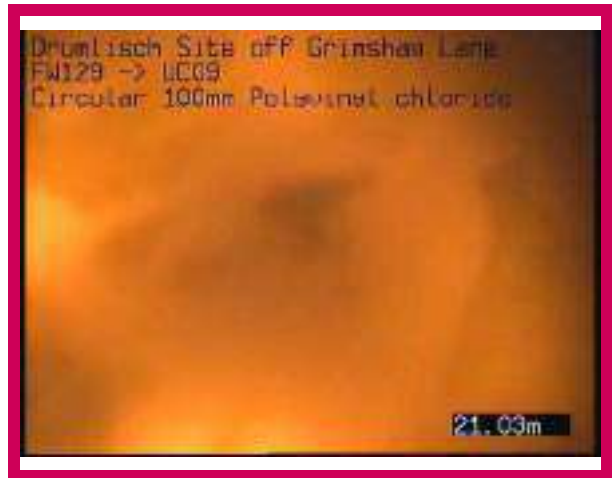
2, 00:01:32, 21.03 m Finish node, major connection without manhole, reference: UC09
