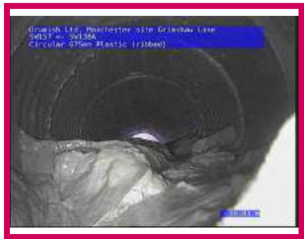
2, 00:02:45, 36.82 m Finish node, manhole, reference: SW138A, Rubble in buried chamber
