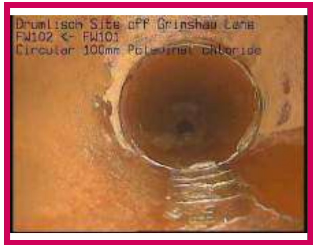
2, 00:04:25, 41.45 m Settled deposits, fine, 5% cross-sectional area loss
