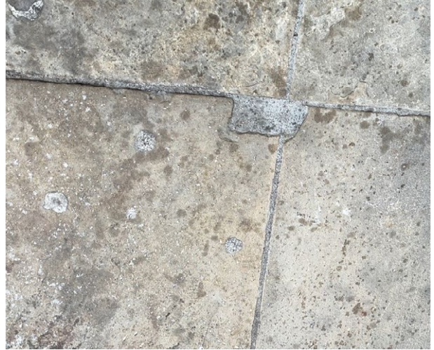
Figure 10: Image showing damage and spalling to existing colonnade paving units
