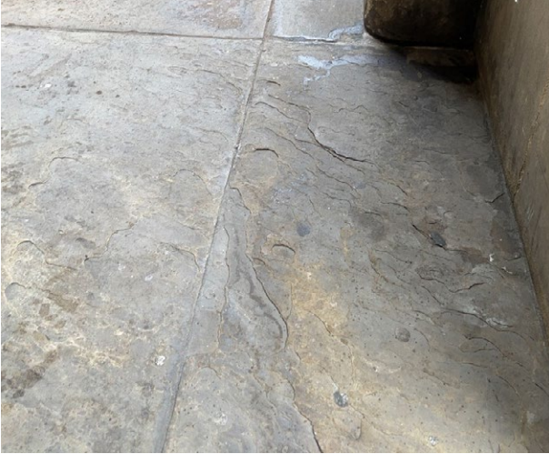
Figure 9: Image showing damage and spalling to existing colonnade paving units
