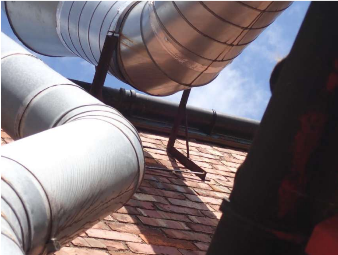
Photograph 7 – View of the pipes for the HVAC system coming out of the wall of Section 2.
