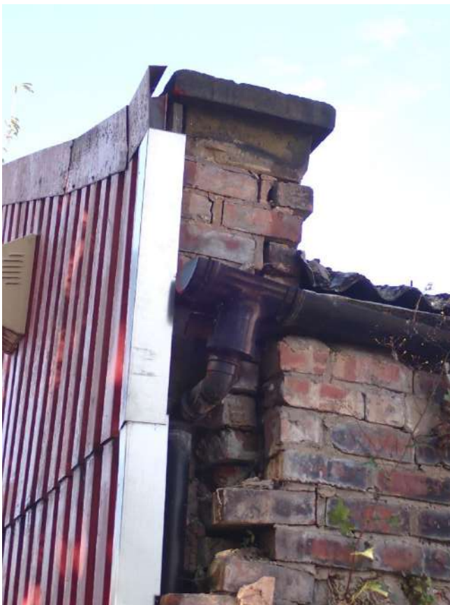
Photograph 8 – View of the PRF formed by damaged brickwork at the southwestern corner of Section 2.
