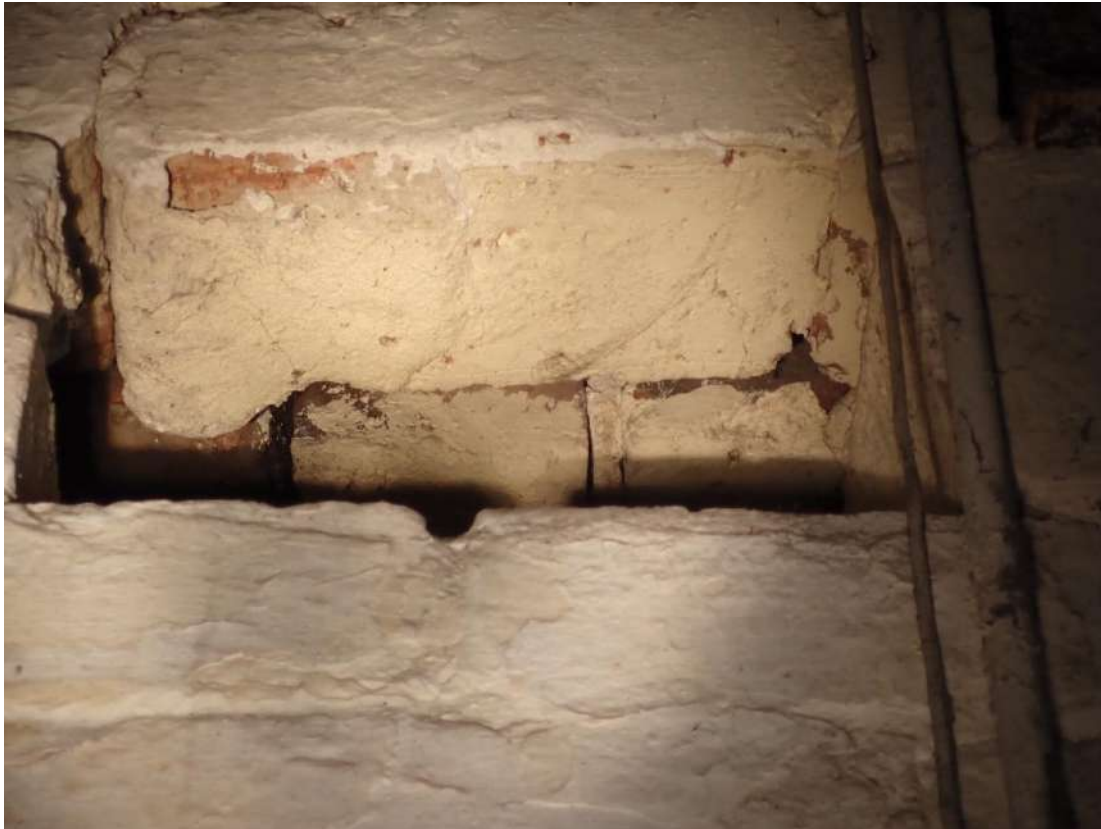
Photograph 15 – View of a gap in the brickwork forming a PRF in the wall of Section 2.
