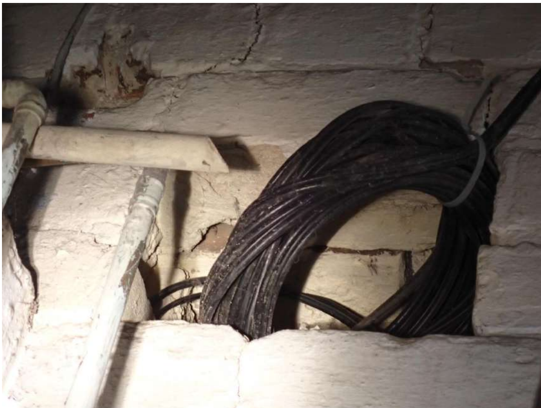
Photograph 16 – View of a PRF formed by a missing brick in the wall of Section 2.
