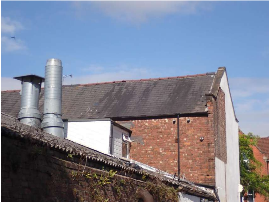
Photograph 3 – View of the western aspect of the building showing the missing mortar from the ridge tiles and the raised tiles.
