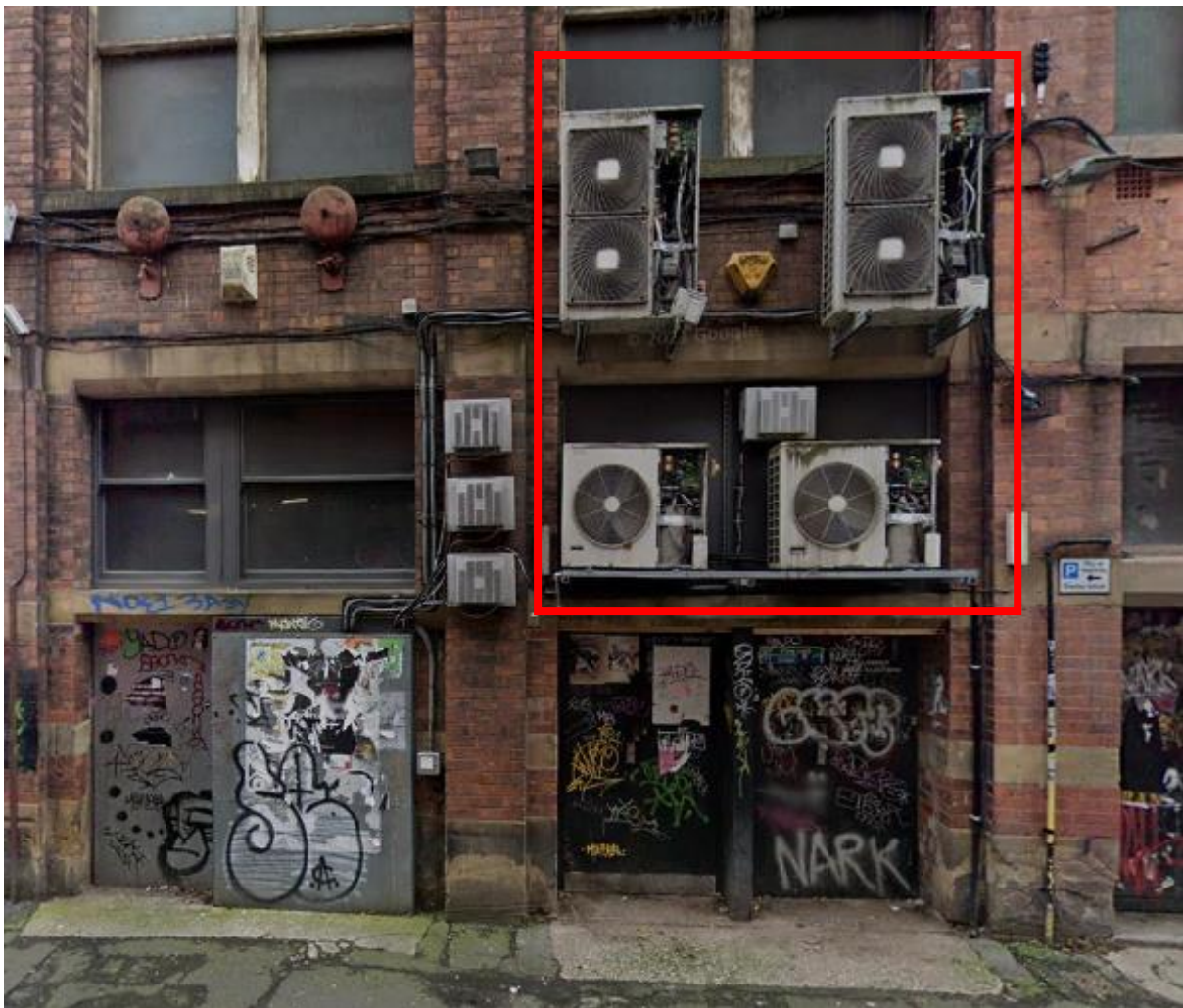
Figure 9 Former condenser unit positions on Spear Street.
