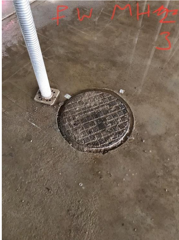
13. P2 FW MH3 – Manhole lid could not be lifted
