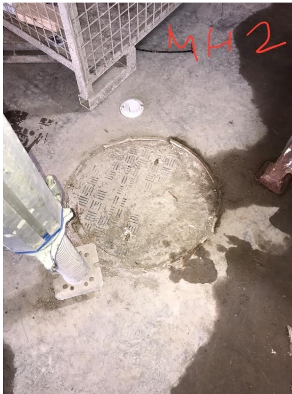
12. P2 FW MH2 – Manhole lid could not be lifted
