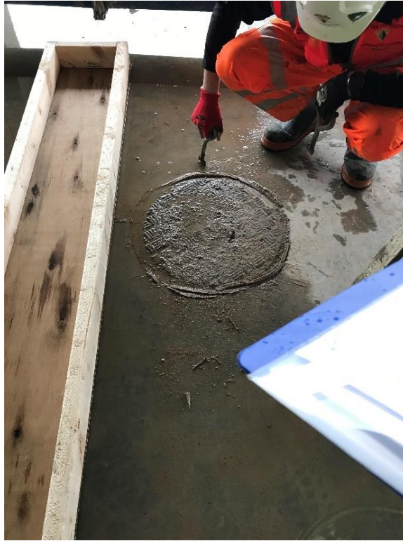
11. P2 FW MH4 – Manhole lid could not be lifted
