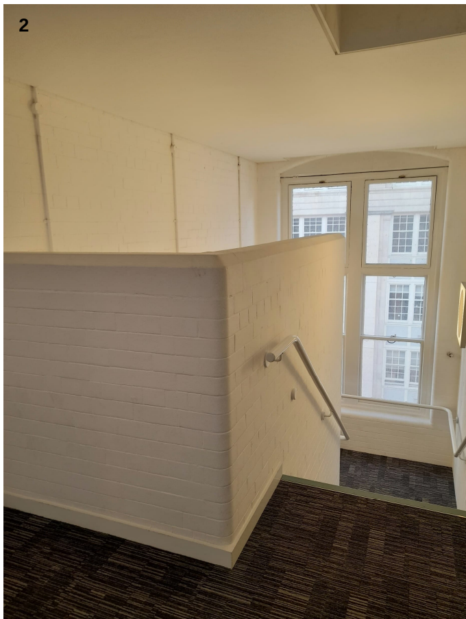
Exposed painted brickwork at the top of the rear staircase
