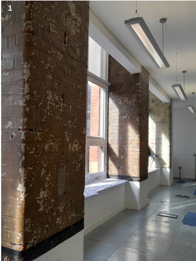
Exposed painted brickwork
