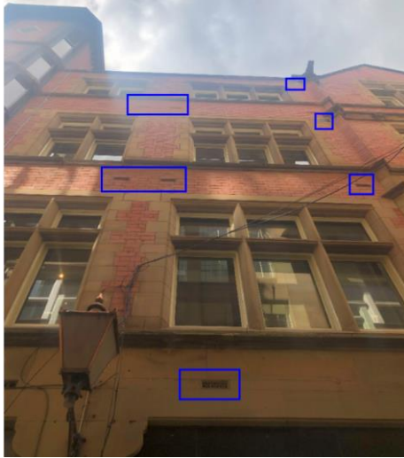
Figure 3 Photographs showing visible MVHR terminations at position 'Y'
