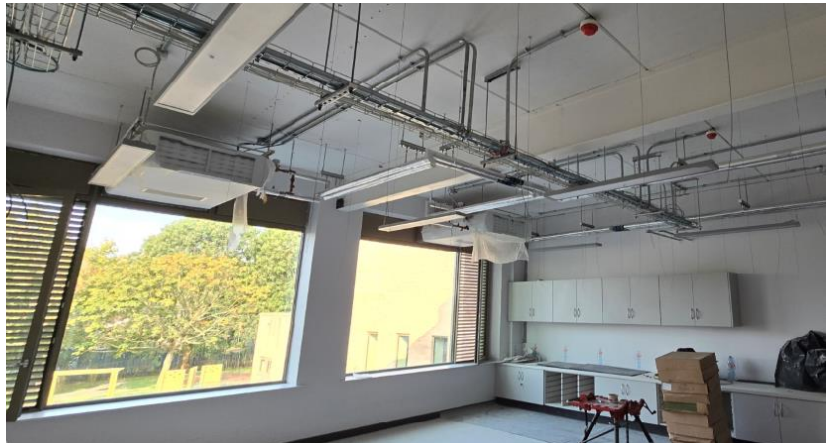
Figure 3: Monodraught hybrid ventilation Installation with purge ventilation openings
