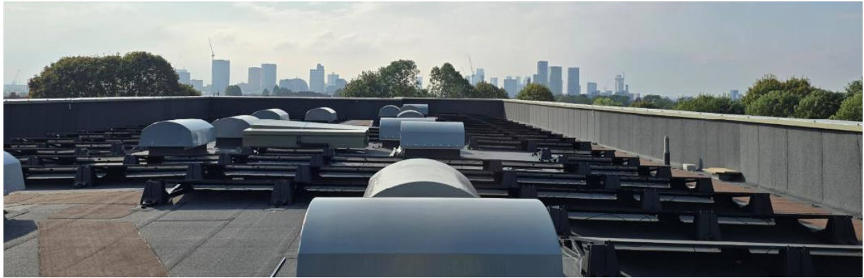
Figure 1: PV installation on the main school roof, along with Monodraught actuated roof cowl ventilation stack terminals.
