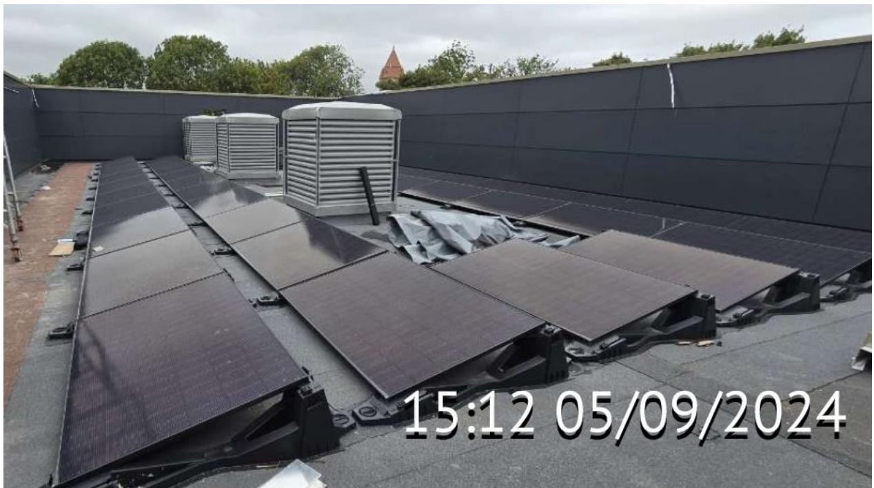
Figure 2: PV installation on the hall roof, along with Monodraught windcatcher Zero terminals.
