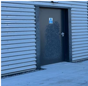
3.10 (C) Personnel Access/Escape Door Set- Warehouse, steel escape doors in PPC Finish Anthracite (RAL 7016)
