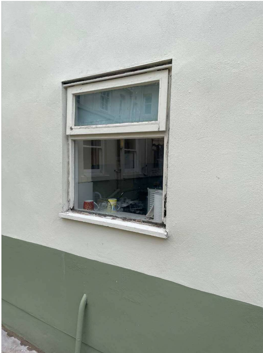
Photo 2. Casement window requiring replacement.
