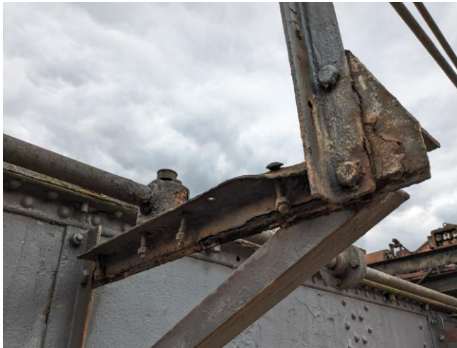
Figure 2-29 Crane beam balustrade – corrosion & deformation
