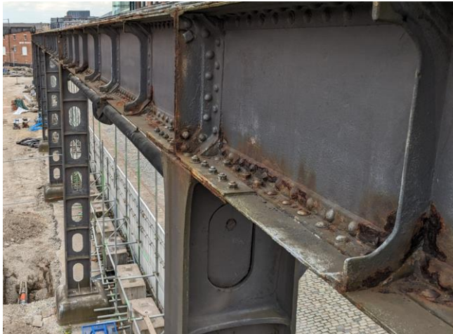
Figure 2-38 Typical corrosion to Gantry beam
