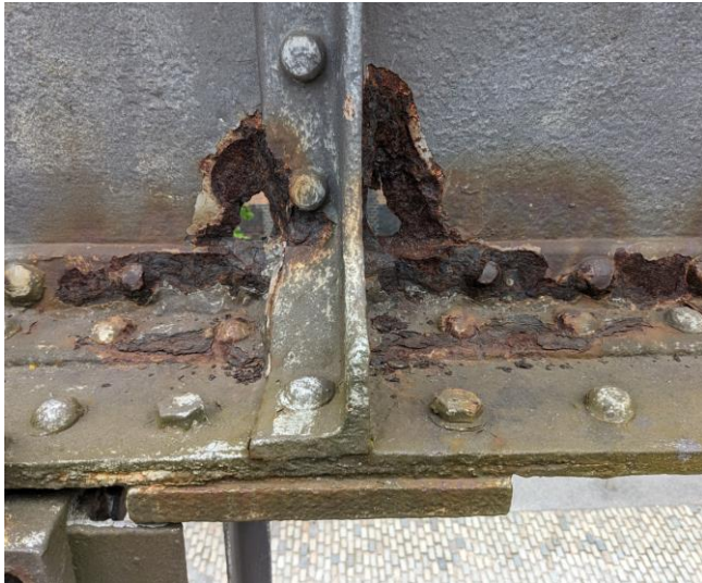
Figure 2-37 Severe corrosion to Gantry beam at stiffener
