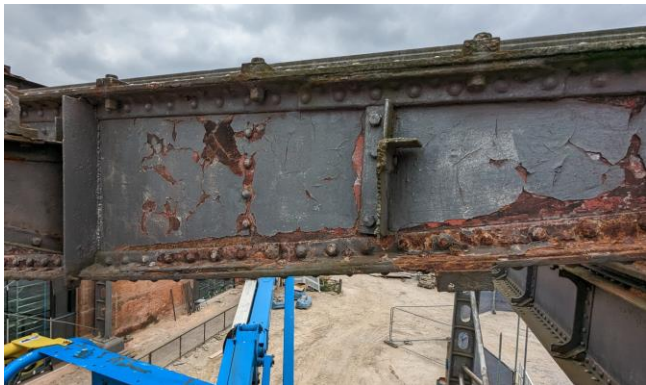
Figure 2-24 Corrosion to side face crane beam (western)
