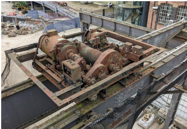
Figure 2-30 Lifting gear to western crane beam
