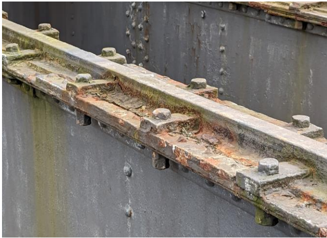
Figure 2-23 Corrosion top face crane beam
