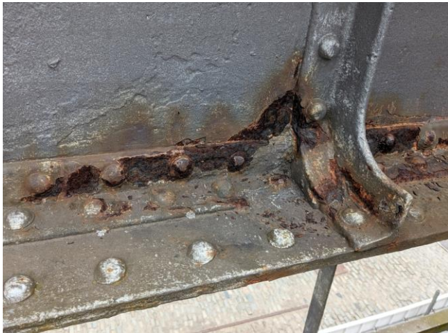
Figure 2-36 Typical corrosion to Gantry beam at stiffener
