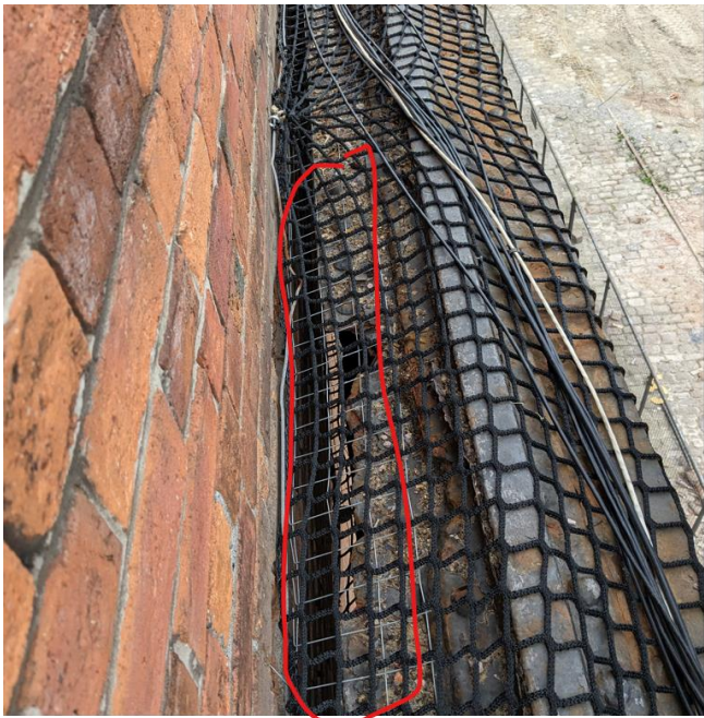
Figure 2-33 Severe corrosion & loss of section width – southern face of south Gantry beam, top flange
