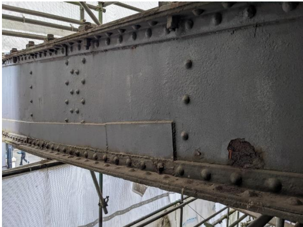
Figure 2-28 – Previous repair to crane beam
