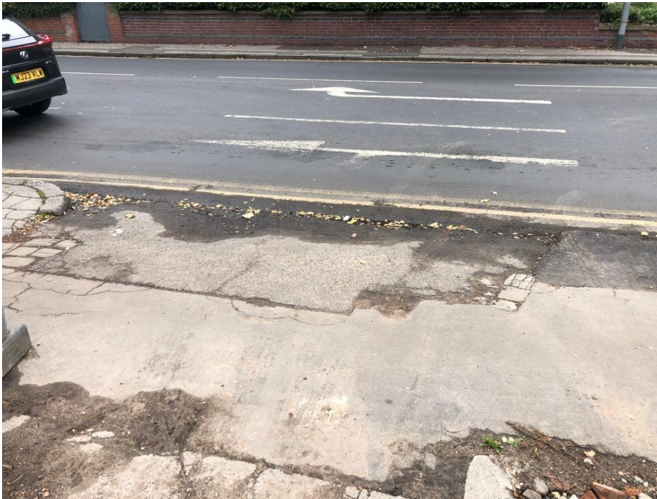
Fig.1 – Existing tarmacadam footpath in state of disrepair. Tarmacadam patch repairs are failing exposing cobbled footway beneath.
