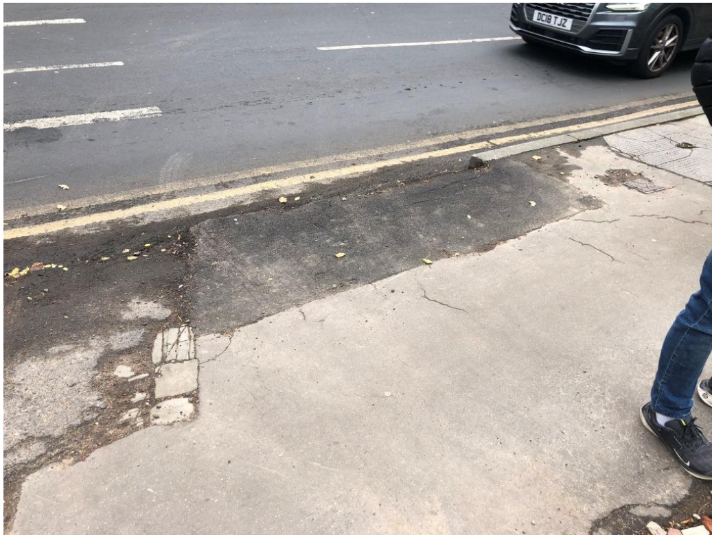
Fig. 3 – Existing tarmacadam footpath in state of disrepair. Concrete kerbs appear to be absent. Existing cobbles are showing through subsequent tarmacadam repair.
