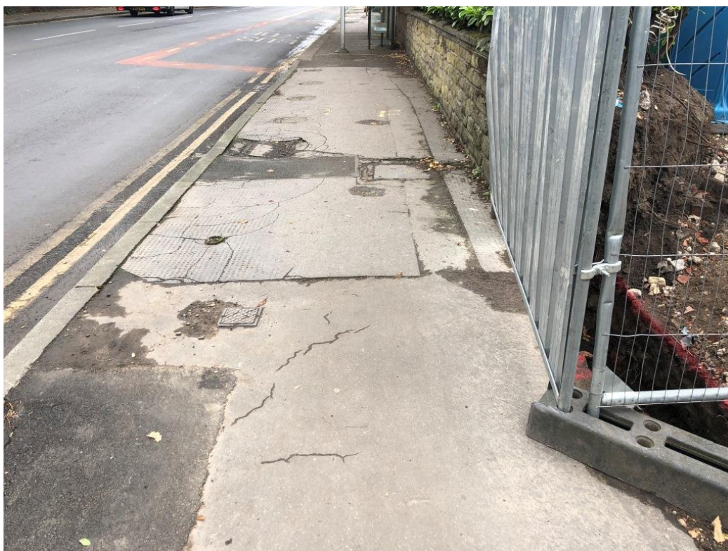
Fig. 4 – Evidence of crazing and previous repairs to tarmacadam surfacing. Footpath terminates at site boundary wall.
