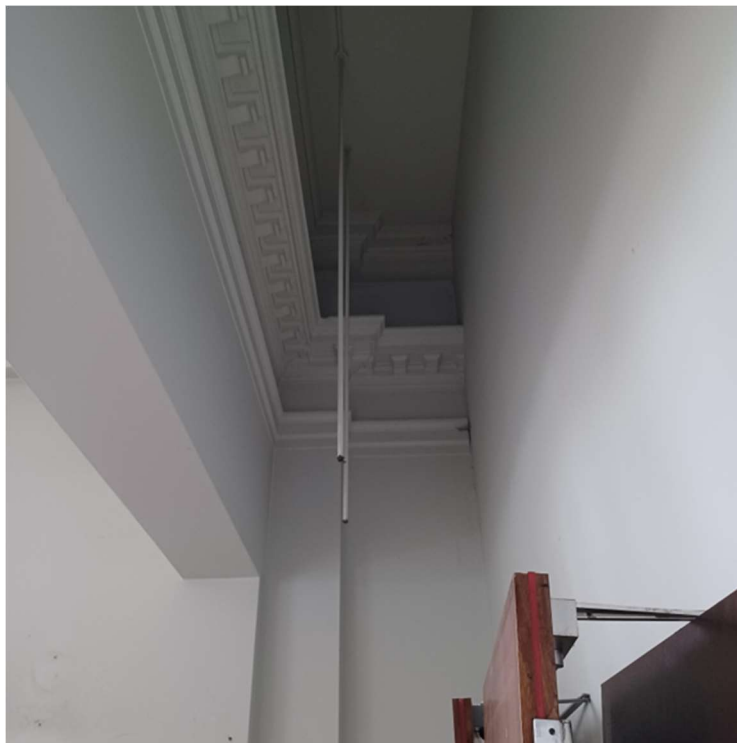
Recess between the arch and partition wall. Note the cornice remains undamaged.
