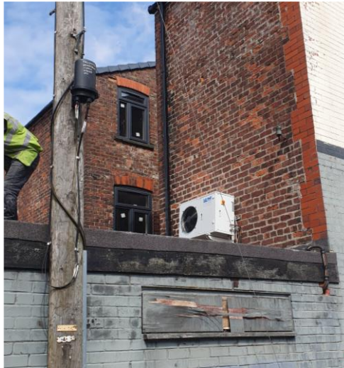
Figure 10 Location of the external condenser unit
