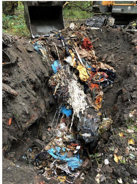
Figure 4. Example area coverage by visually hazardous materials that would not be supportive of ceasing the excavation
