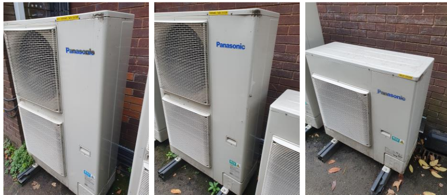
Figure 4 Condenser units' location
