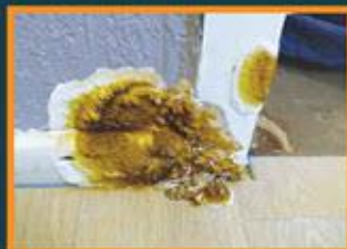
Wet & Dry Rot Control
