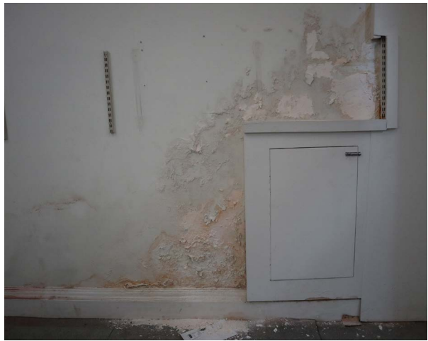
Figure 19 Photograph showing damaged plaster to east corner
