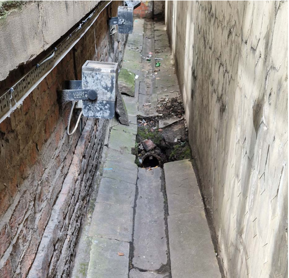
Figure 24 Photograph showing cracked paving slabs and broken out gully
