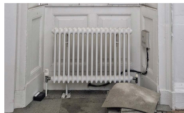
Figure 21 Photograph showing existing modern radiators
