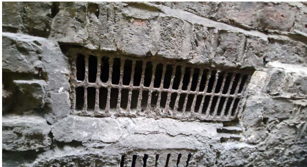
Figure 22 Photograph of existing historic corroded cast iron vent cover (photo shows the only remaining intact cover)
