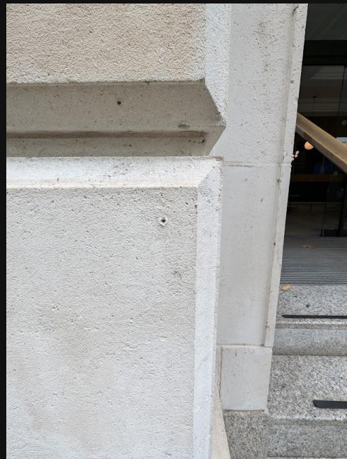
Existing holes in front stonework where signage has been relocated in the past – we propose to reuse these fixing points and make good where items relocated.
