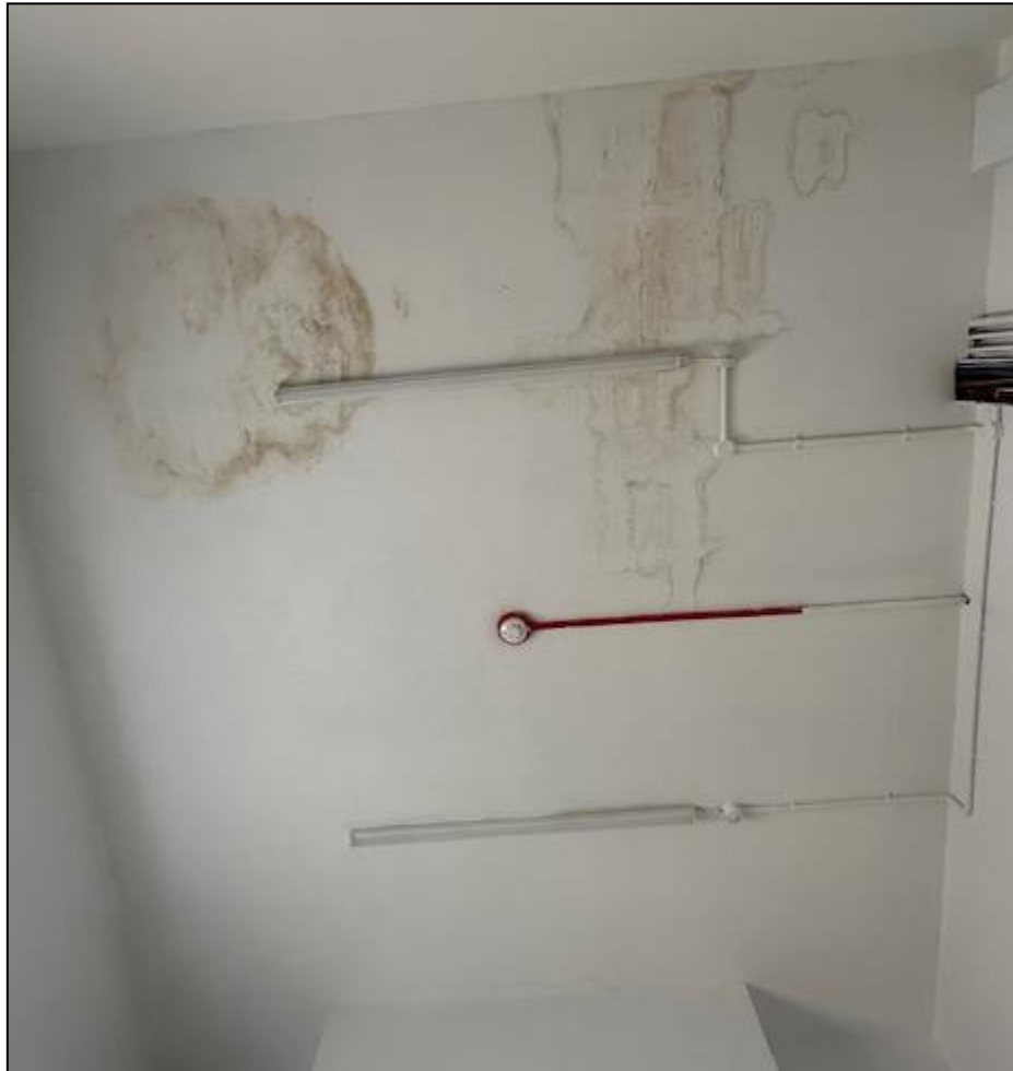
Figure 2. Water damaged ceiling to classroom SG11.
