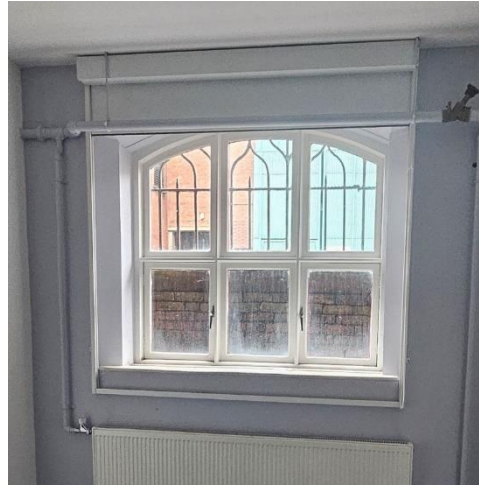
Example of blackout blinds installed in B.003
