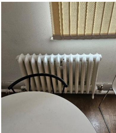
Existing cast iron radiators to be redecorated in Hammerite Paint – White Satin Halliday Meecham Architects
