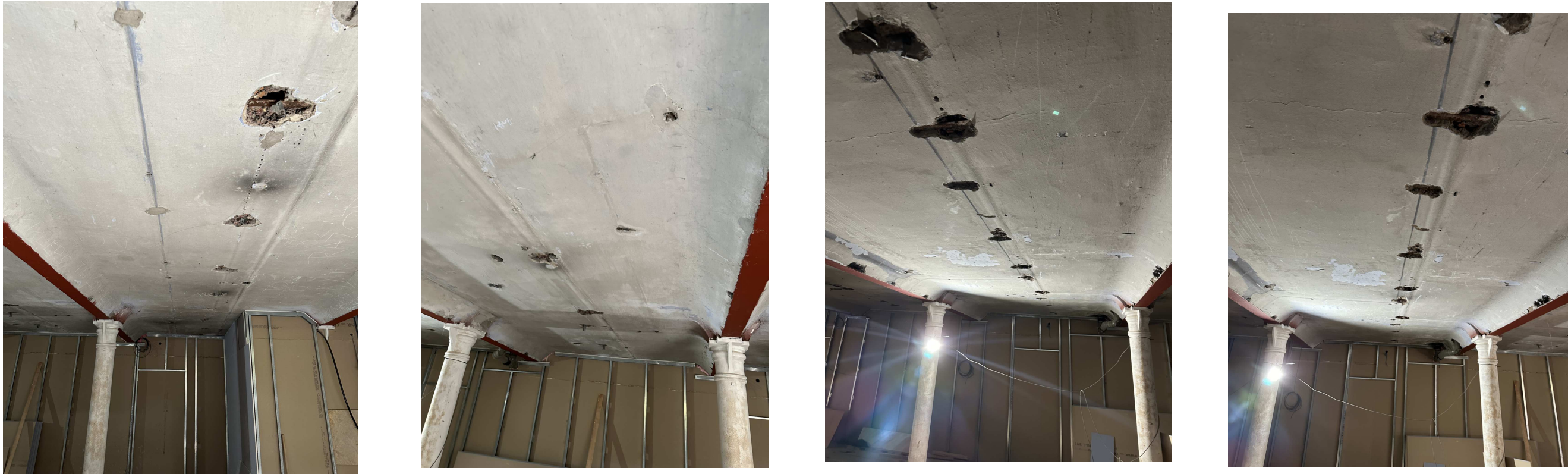
Typical damage to the existing ceiling finish
