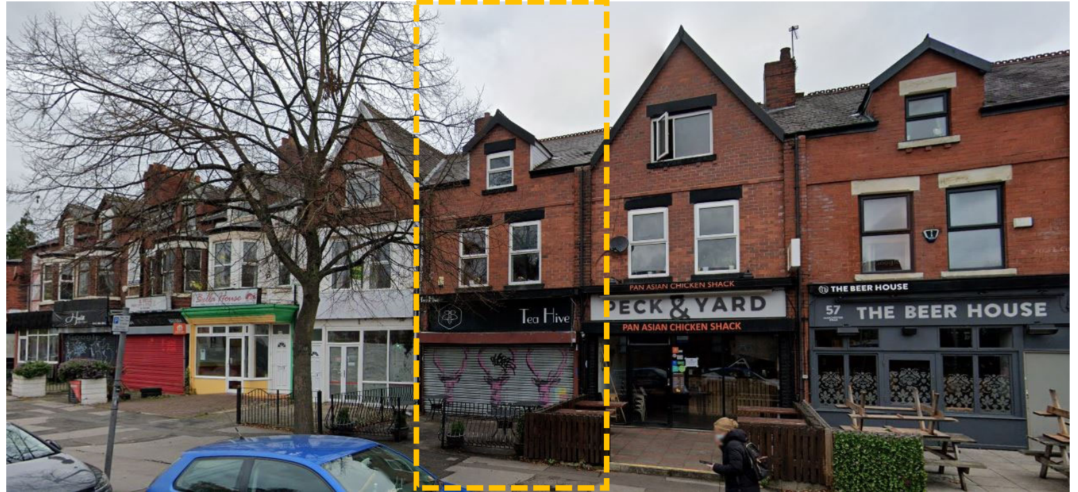
Front Façade in need of repair
