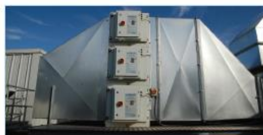
3 ESP Units Stacked in modular formation
