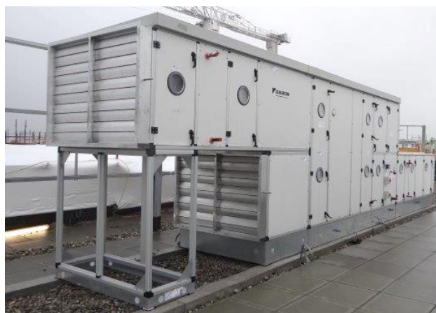
Example of a Roof Level Kitchen Air Handling Unit
